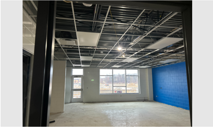
Description Zone F classroom with ceiling grid light fixtures
