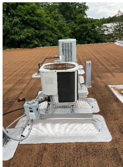
Mill Lake School Complex – Split System
