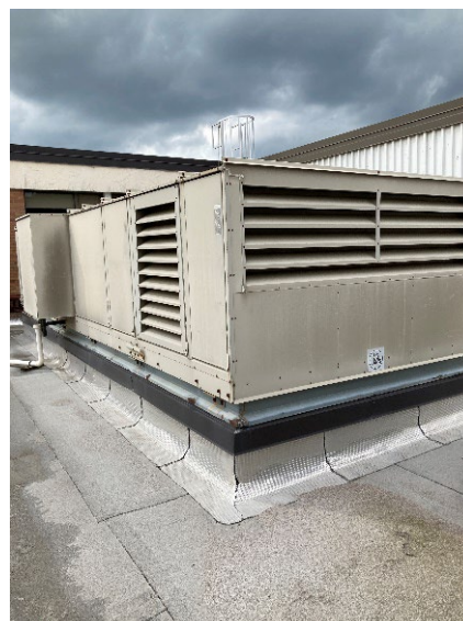
Monroe Twp. Middle School - AHU
