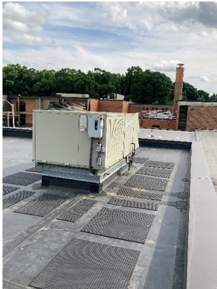
Monroe Twp. Middle School - RTU
