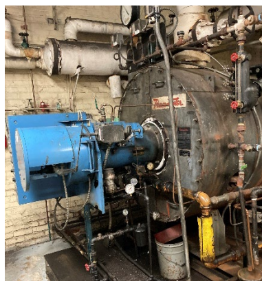
Applegarth School – Steam Boiler
