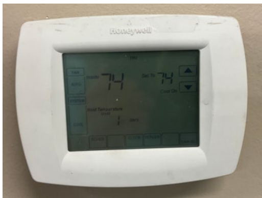
Programmable Thermostat (AHU)
