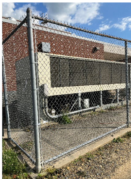
Barclay Brook School – Chiller
