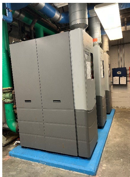
Barclay Brook School - Boilers
