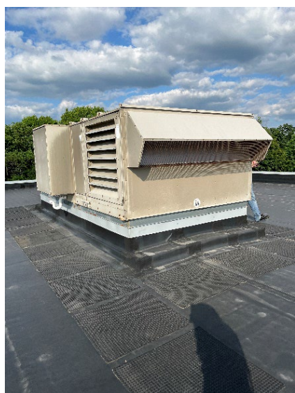
Barclay Brook School - AHU
