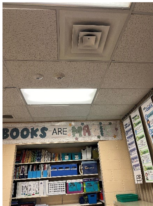
Lighting at Brookside School
