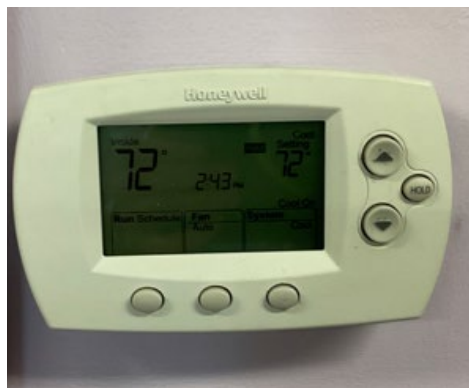
Programmable Thermostat (AHU)
