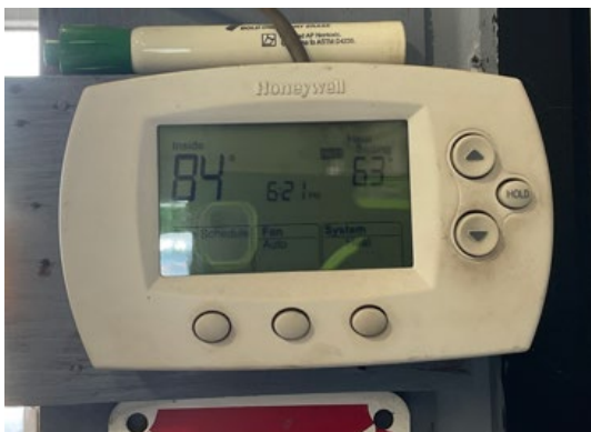
Garage Thermostat (AHU)
