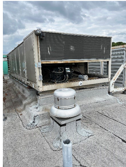
Mill Lake School Complex - RTU
