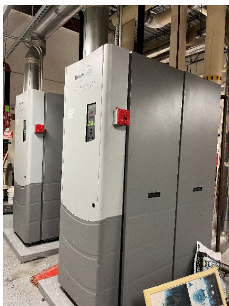
Oak Tree School - Boilers
