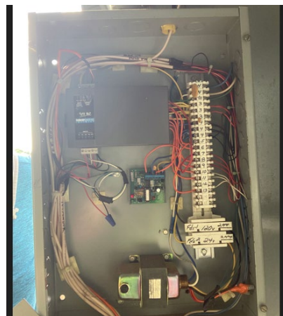
Typical Andover RTU Controller
