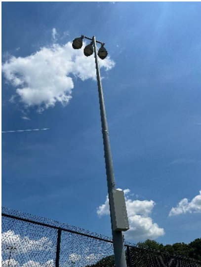
Sports Field - Stadium Lighting
