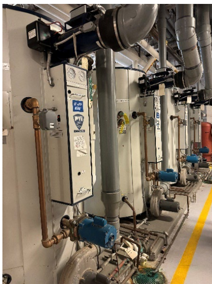
Monroe Twp. High School – Water Heater
