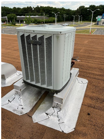
Mill Lake School Complex – Split System
