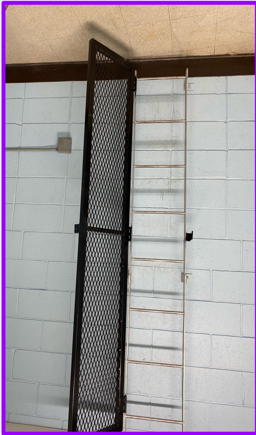
Locking cage over catwalk ladder.
