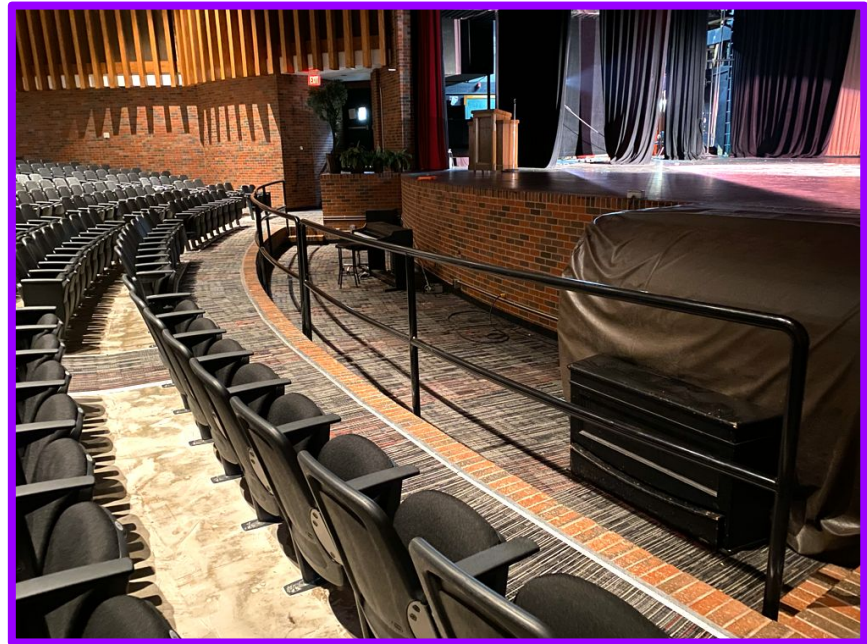
Railing along edge of orchestra pit. It never had one!
