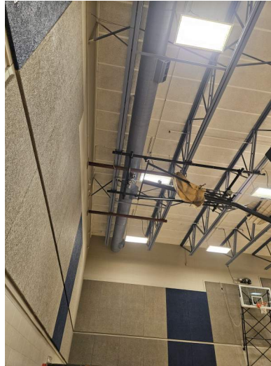
DMS - Wrestling Mat Hoist Support Steel
