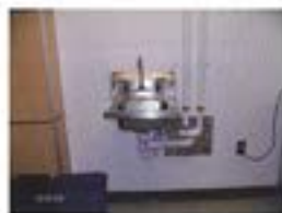
New classroom sink at Bethany
