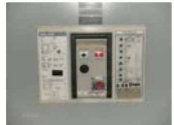
New Main Breaker Settings
