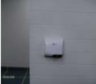
New Restroom Hand Dryers
