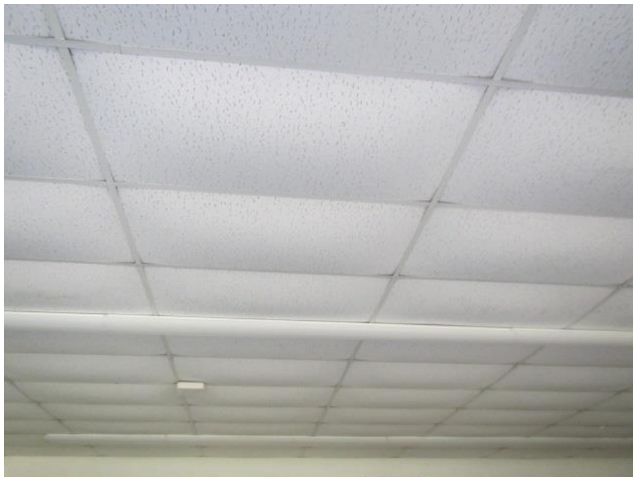
Bowed ceiling tiles in classroom
