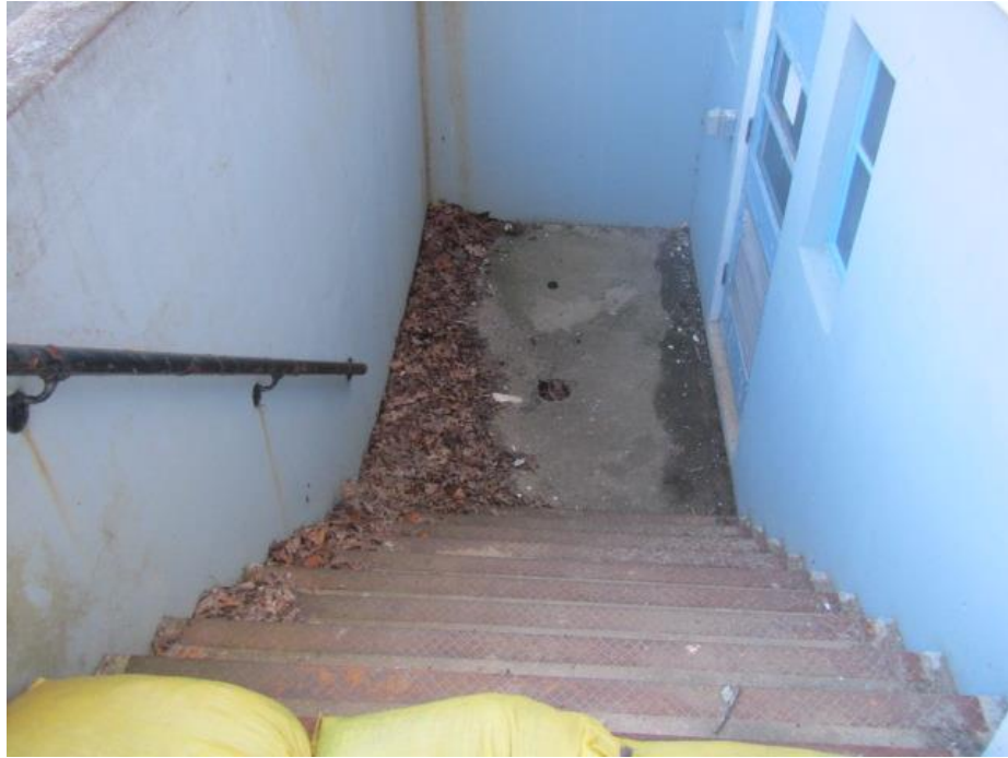
Clogged drain at bottom of boiler room stairwell
