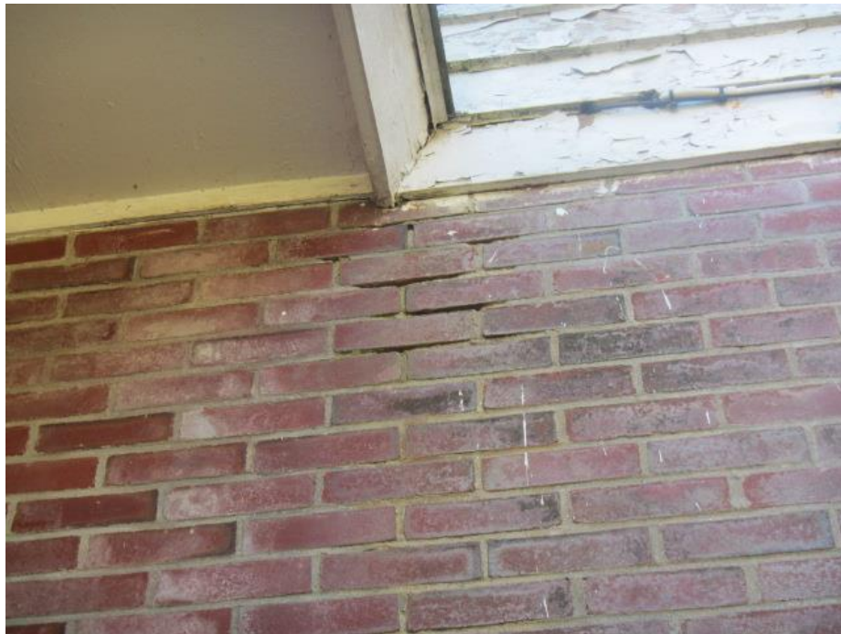
Missing/damaged mortar around exterior brick
