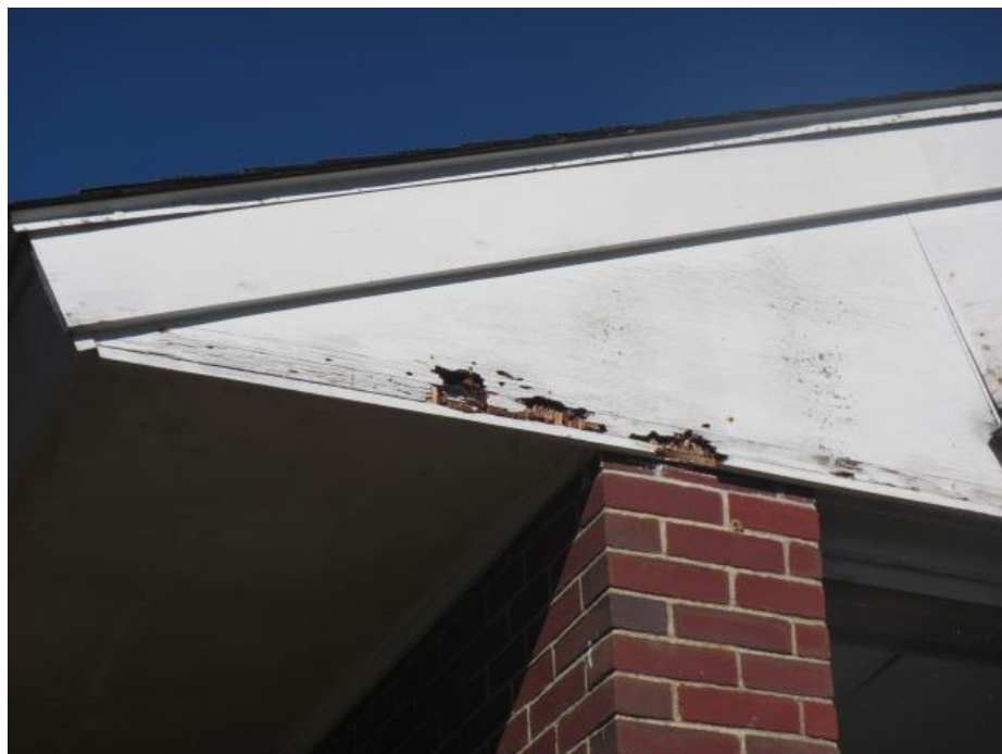
Rotted/delaminating wood along roof
