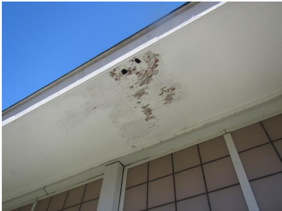
Rotted/delaminating wood along roof
