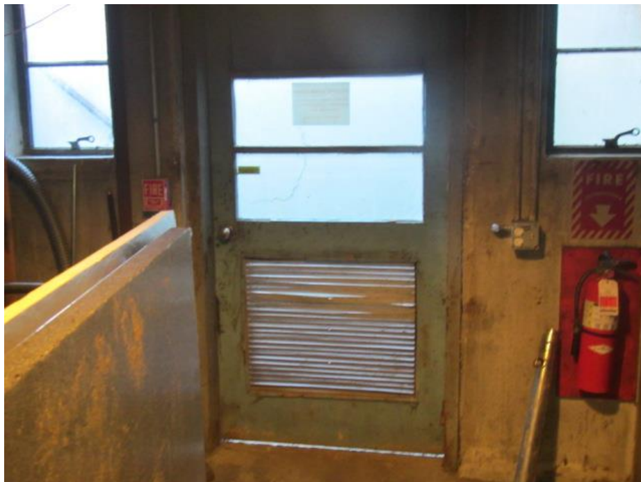
Light penetrating through damaged vent and below exterior door
