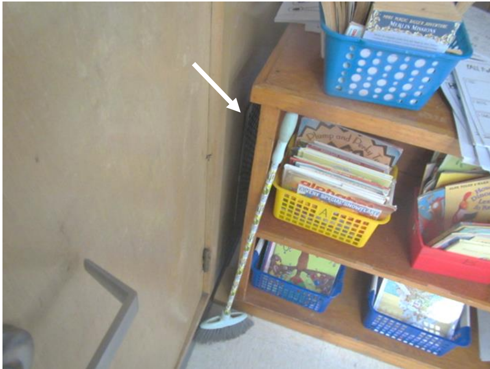
Exhaust vent behind shelf in classroom (arrow)
