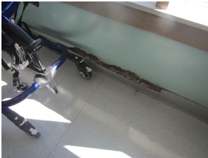
Wall damage in Classroom4 (OT/PT Room)
