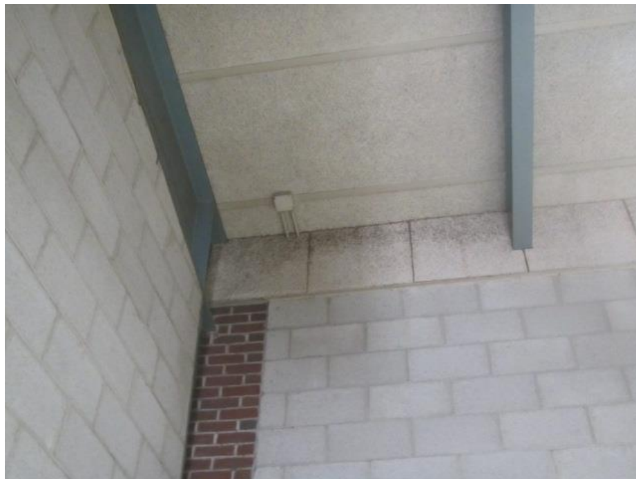
Dark staining on wall panels indicating accumulated dust/debris near ceiling of gymnasium
