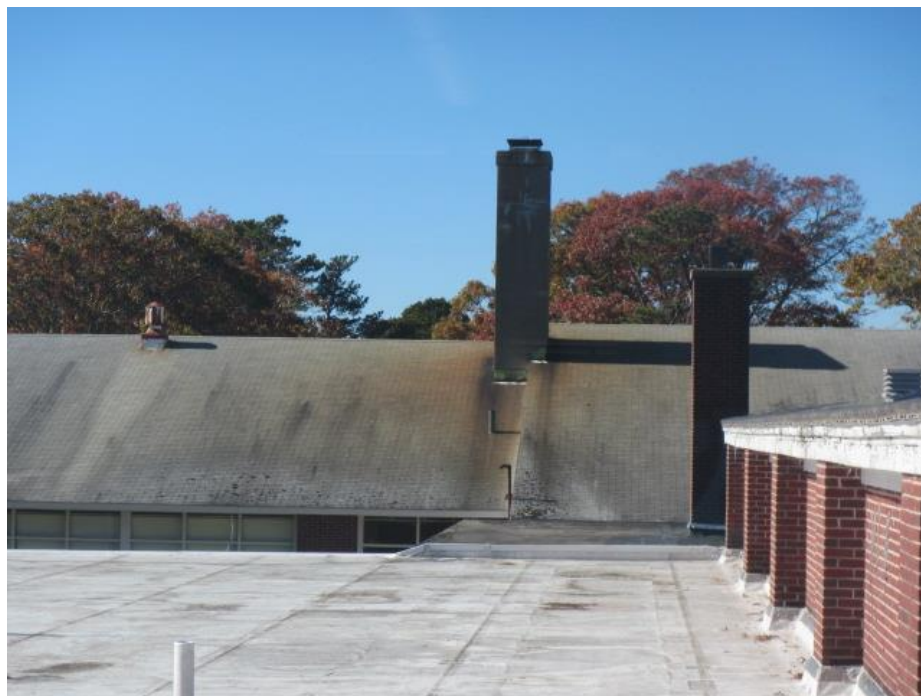
Roof is past its life expectancy and is need of replacement
