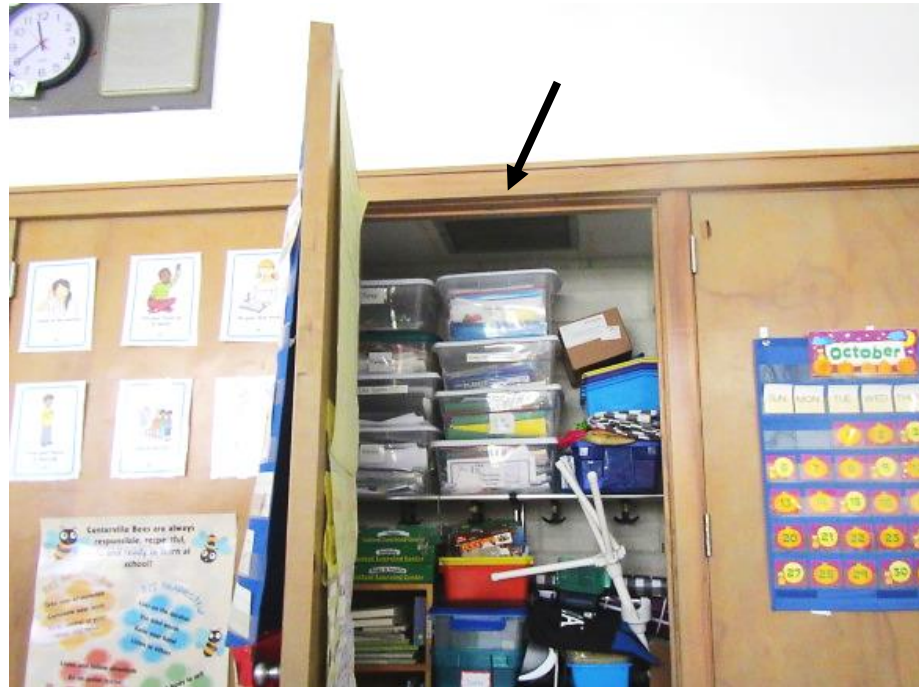
Exhaust vent in the top of coat closet (arrow)
