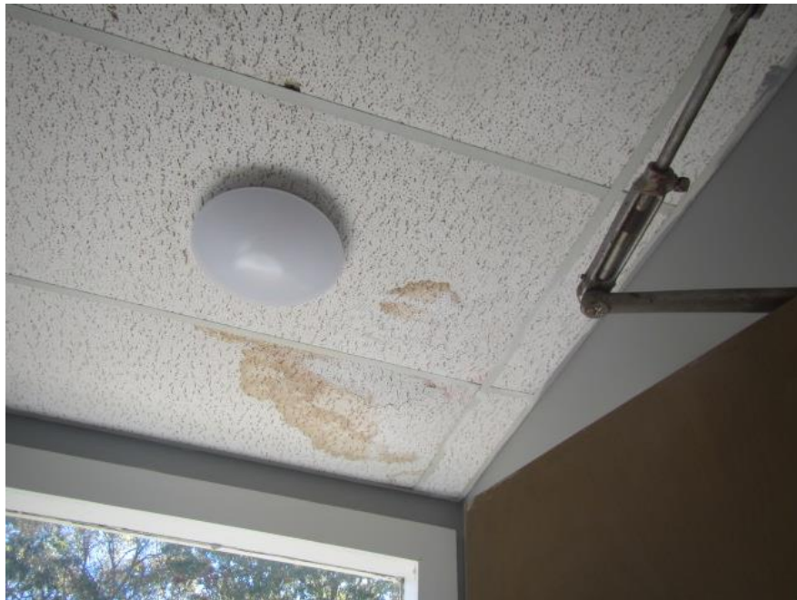
Water-damaged suspended ceiling tile
