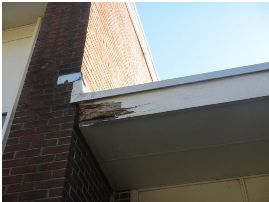
Rotted/delaminating wood along roof
