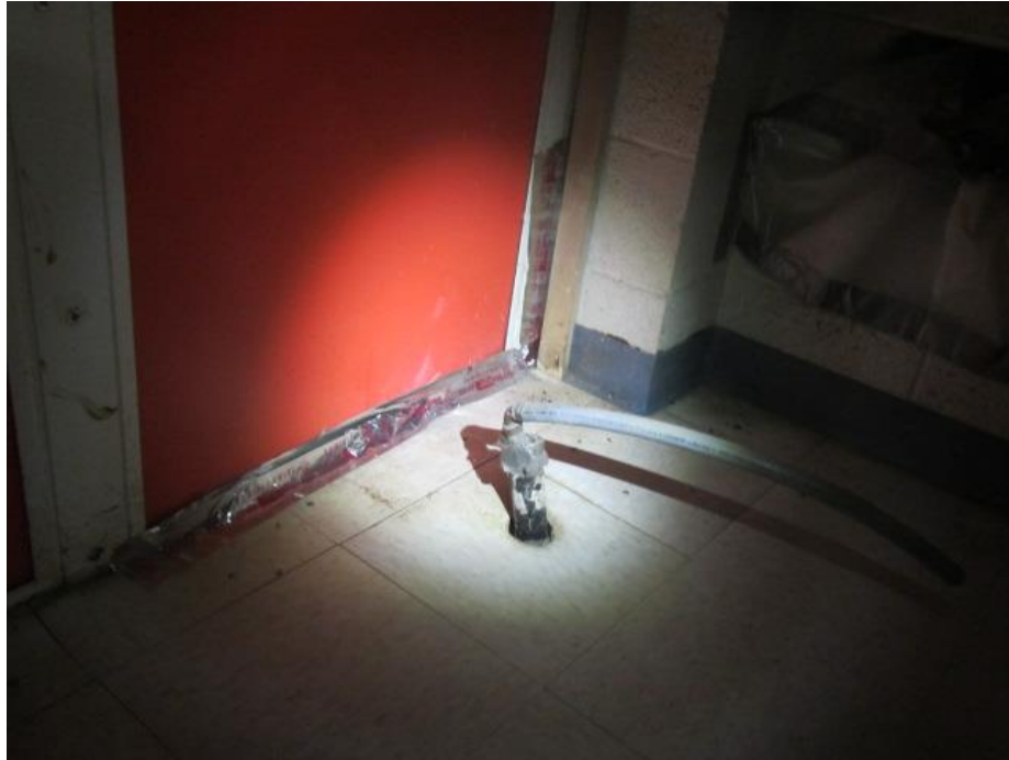
Breach around exterior door under stairwell across from Staff Room
