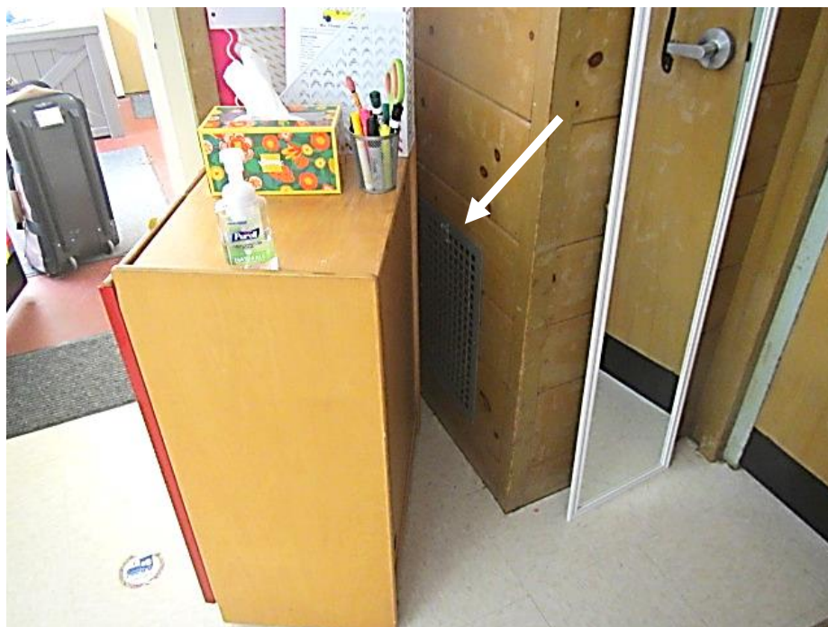
Wall-mounted exhaust vent (arrow) behind bookcase in classroom
