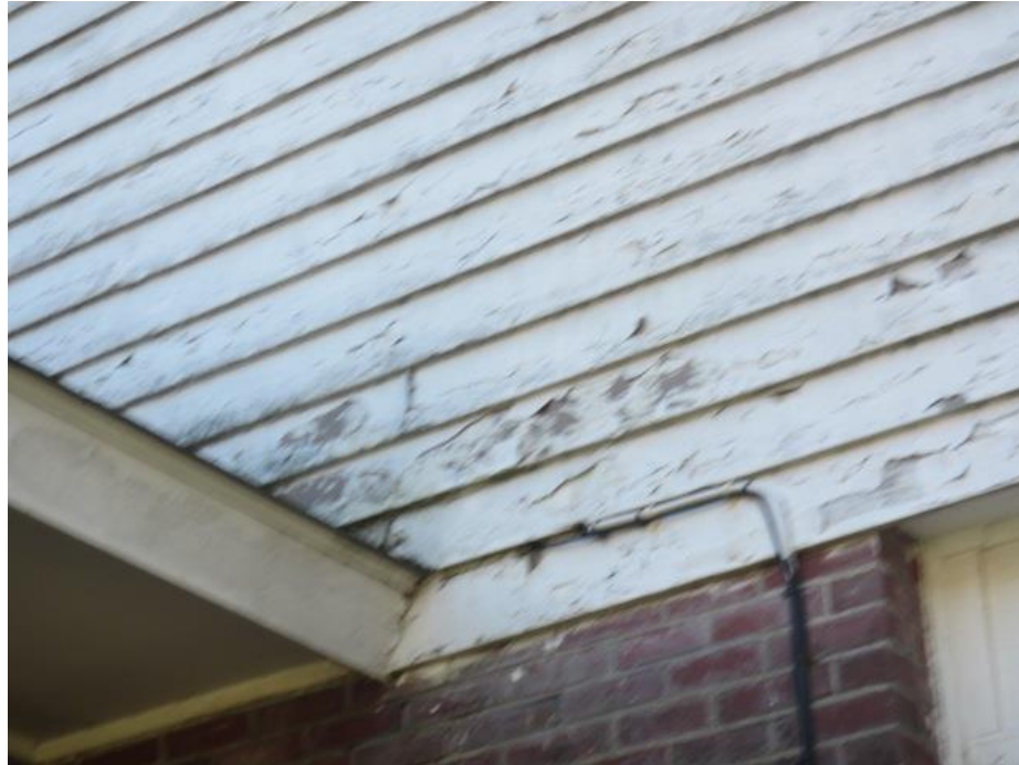
Rotted/delaminating wood along roof/exterior walls
