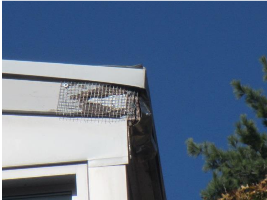
Rotted/delaminating wood along roof
