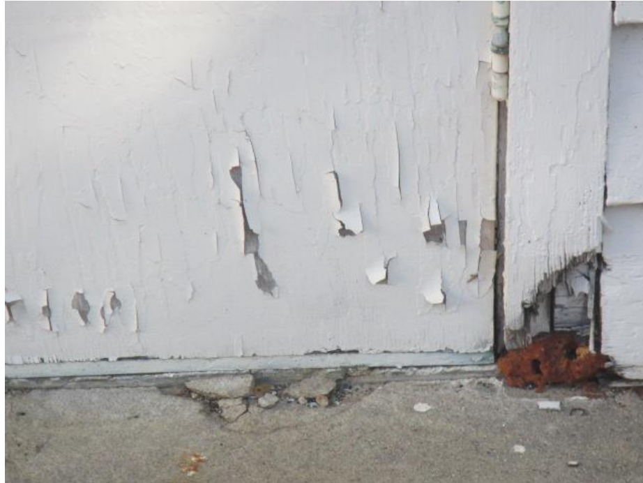
Rotted door frame (filled with foam) and delaminating exterior door
