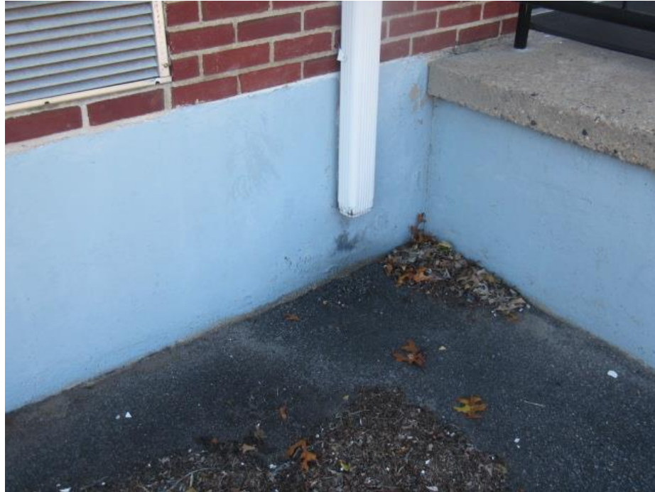
Missing elbow extension at bottom of downspout to drain water away from building
