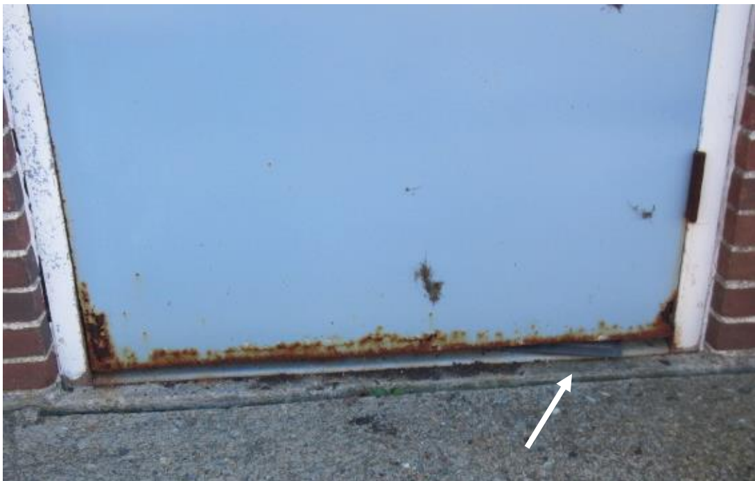
Corroded exterior door, note damaged weatherstripping below (arrow)
