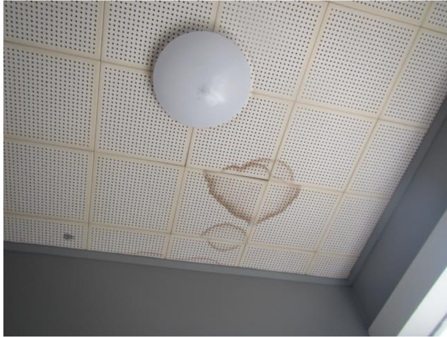
Water-damaged original ceiling tiles adhered directly to ceiling substrate
