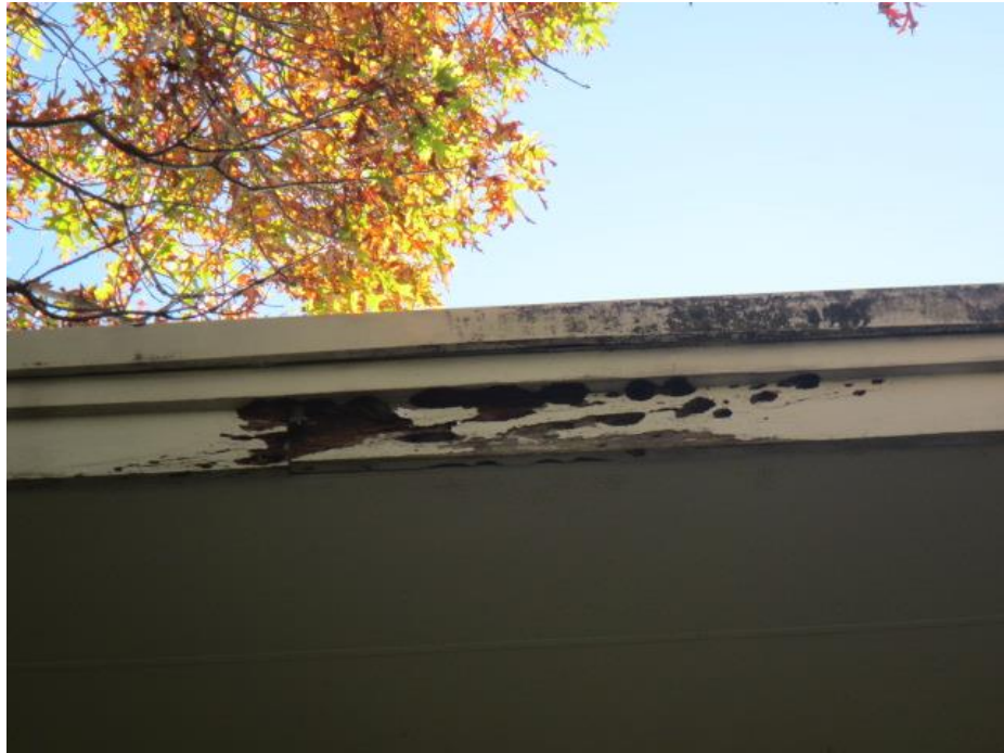
Rotted/delaminating wood along roof
