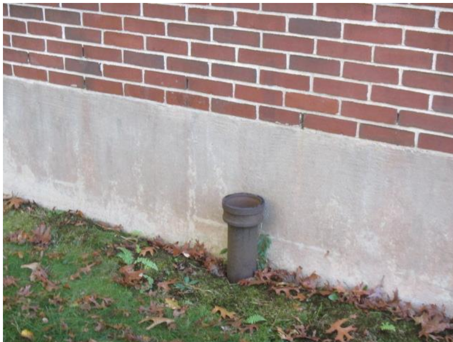
Abandoned drainage pipe for gutter/downspout system
