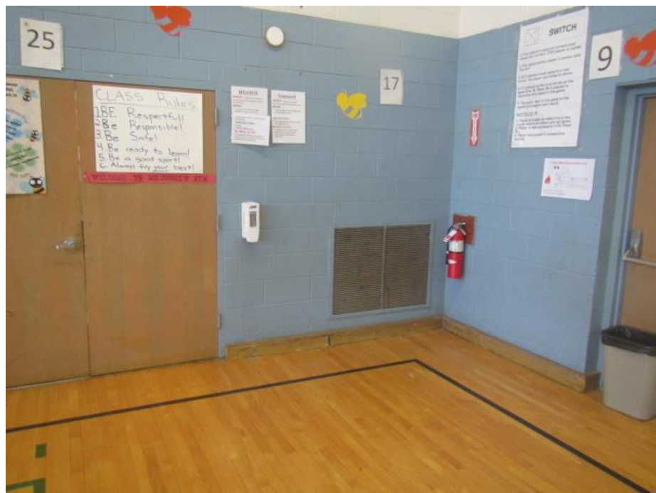
Exhaust vent on wall of Gym across from the AHU
