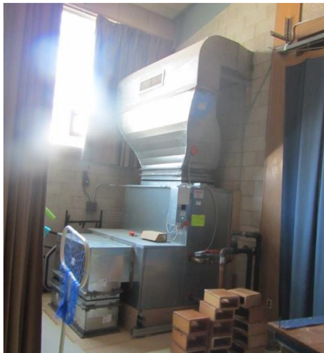
Air handling unit in corner of gymnasium (stage view)
