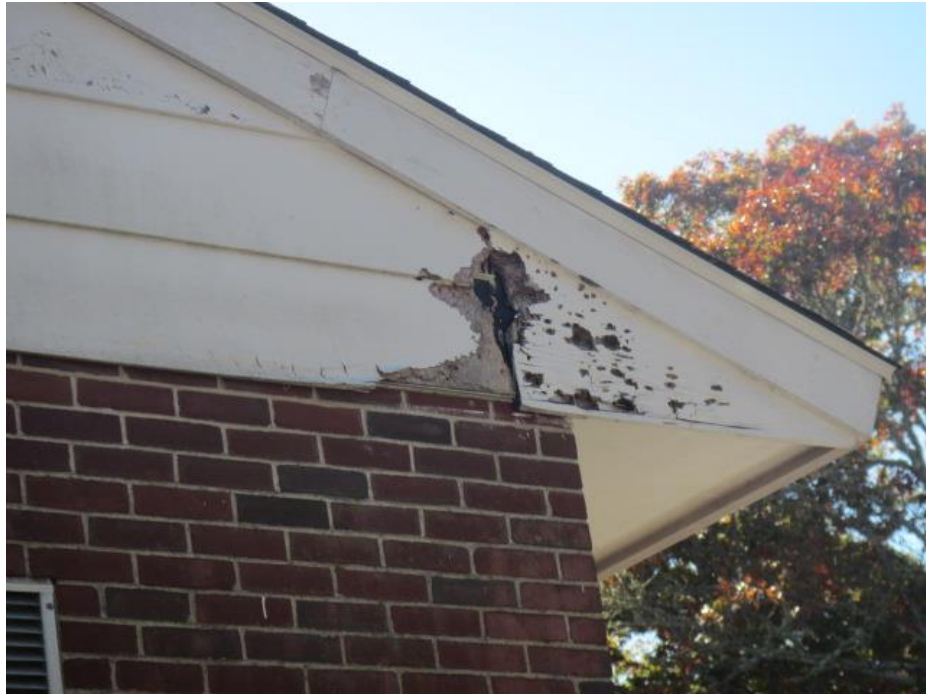
Rotted/delaminating wood along roof
