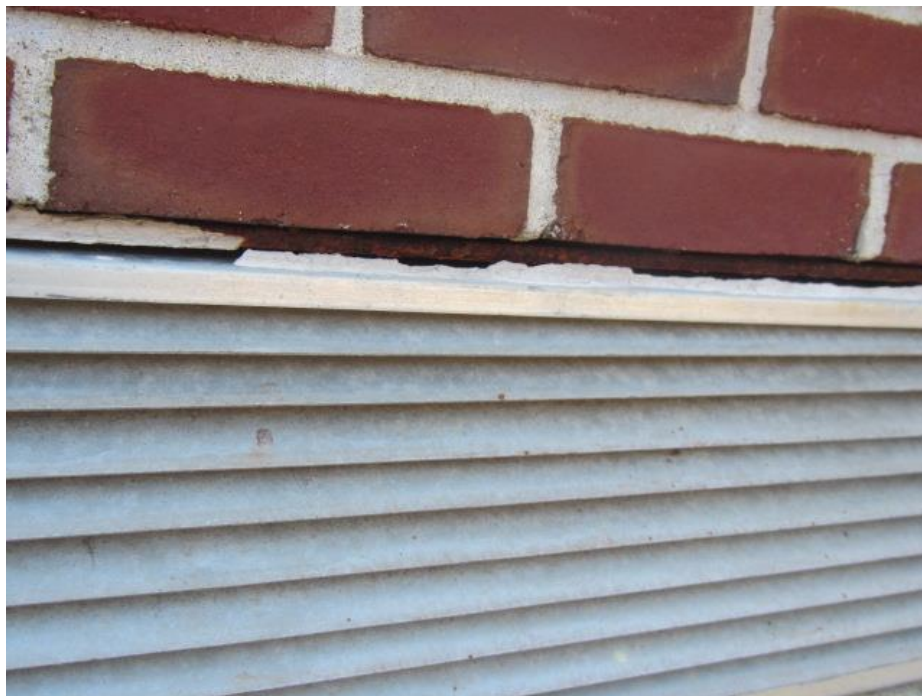
Missing/damaged sealant/caulking around univent fresh air intake
