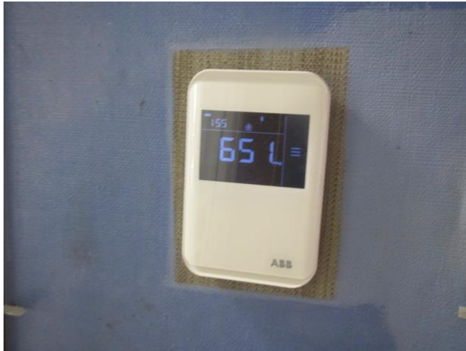
Digital Thermostat displaying carbon dioxide measurement in parts per million
