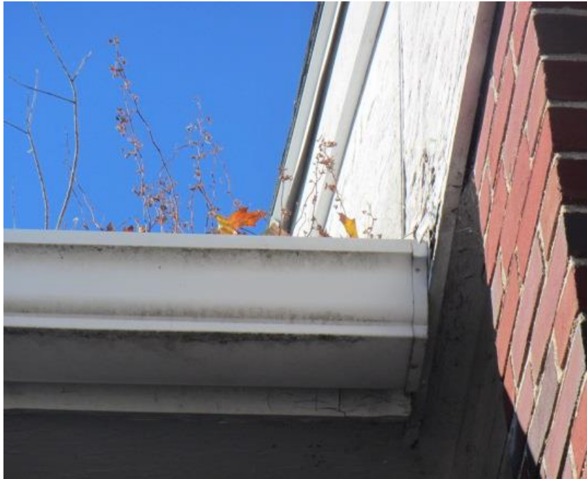
Gutter clogged with debris
