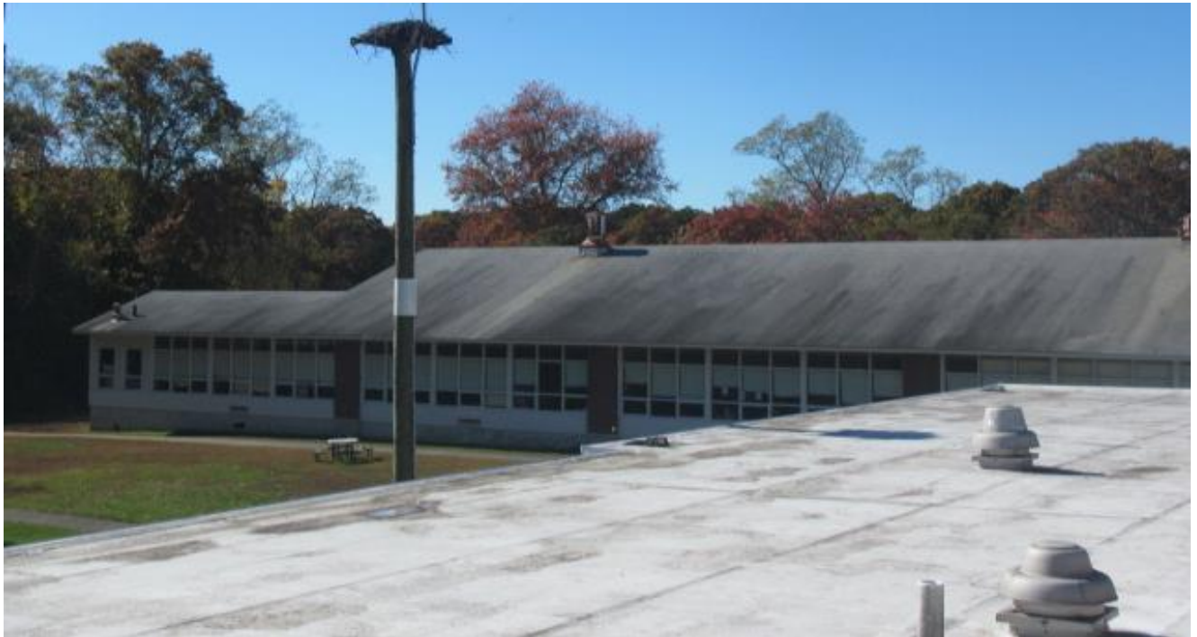
Roof is past its life expectancy and is need of replacement
