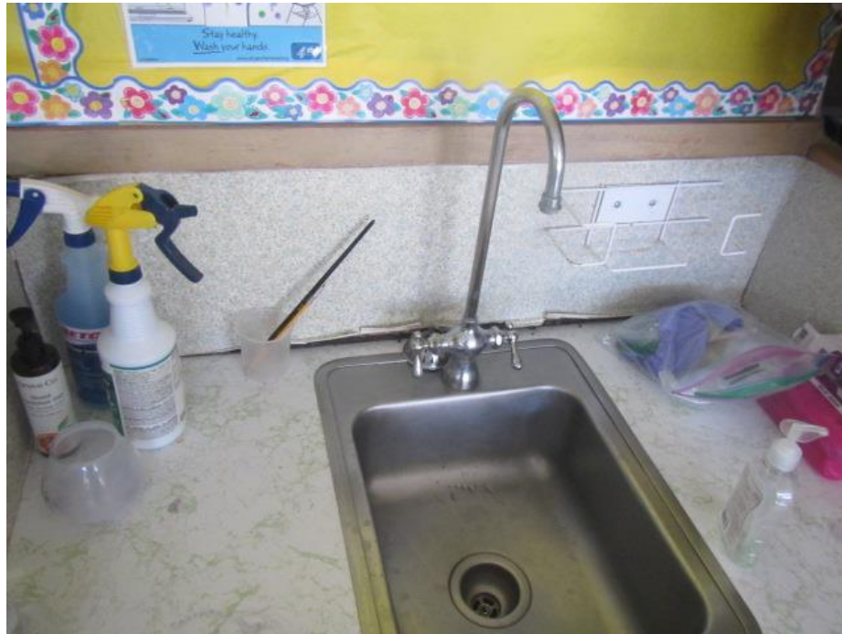
Missing/damaged caulking around sink in Classroom 6
