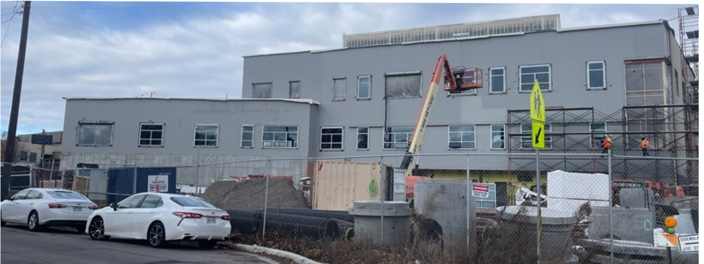
From top left: Bathroom floor tile; installed windows on east elevation; prep for last concrete floor pour; south-side elevation before brick or panels (December 2024)
