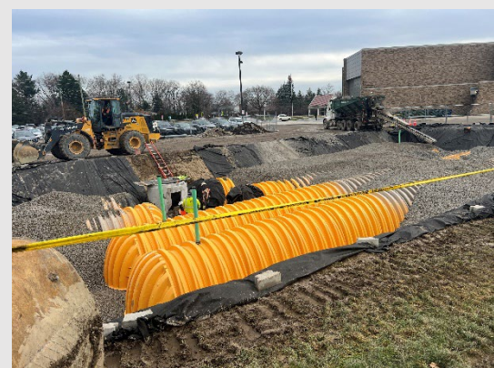
Groves - Underground Detention
