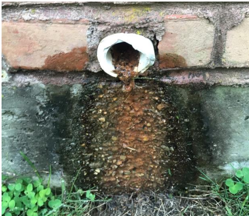
Debris/scale from condensate pipe/drip pans
