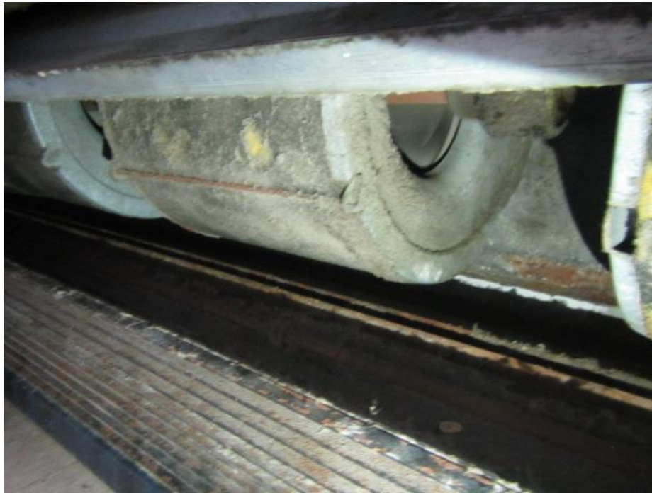
Accumulated dust/debris on interior univent components
