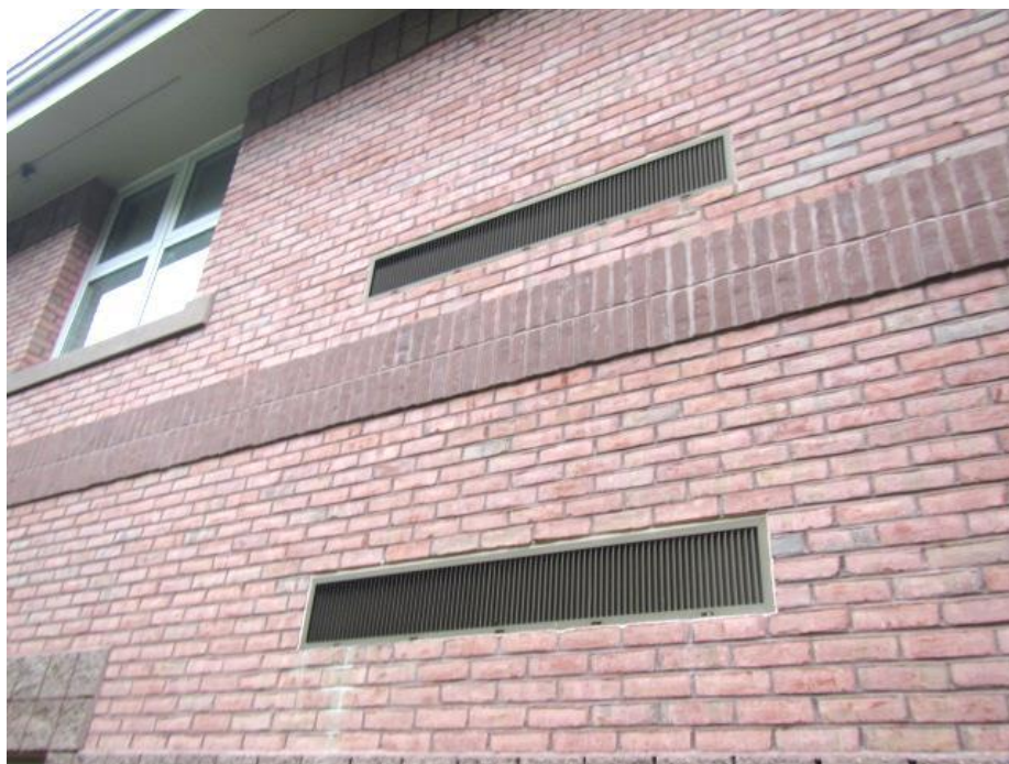
Univent fresh air intakes
