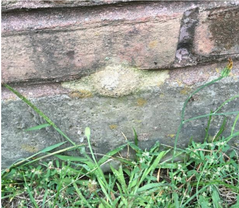
Clogged/plugged weep hole
