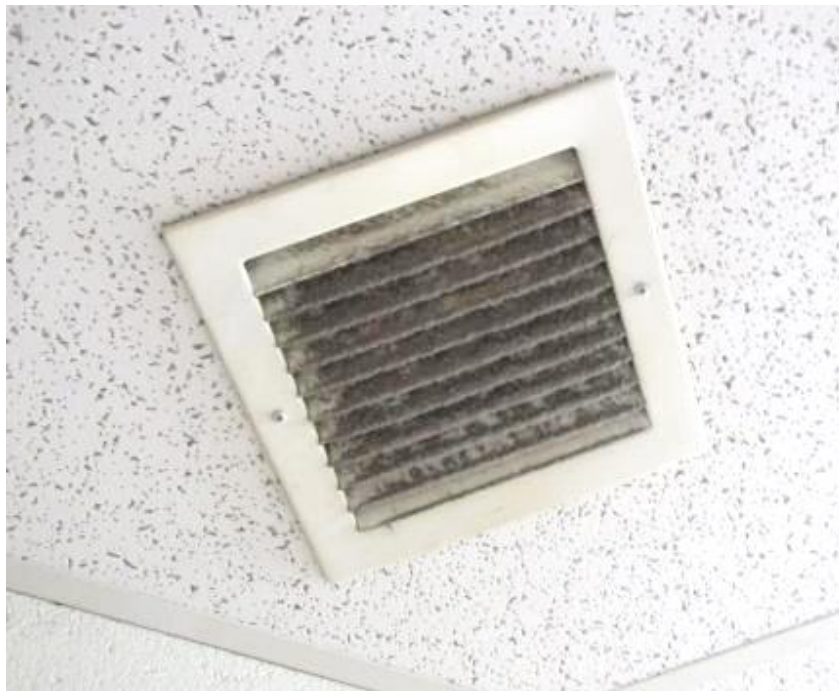
Classroom exhaust vent, note accumulated dust/debris
