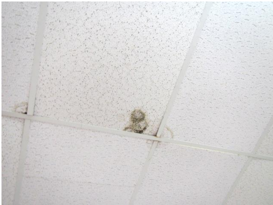
Water-damage/mold growth on ceiling tiles room 219
