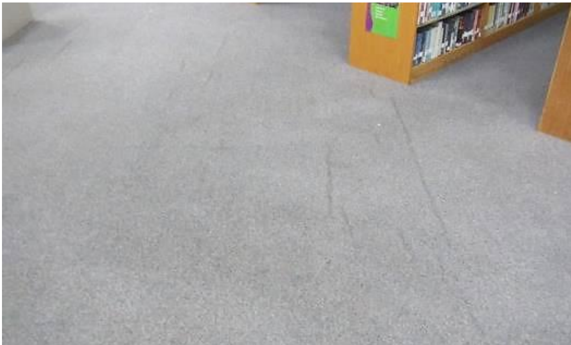
Original (20+ yr.)/wrinkled carpeting in Library
