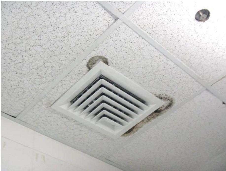
Water-damage/mold growth on ceiling tiles room 107
