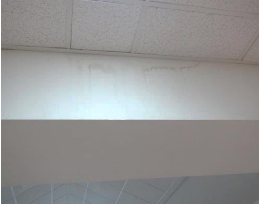
Water-stained gypsum wallboard outside Library
