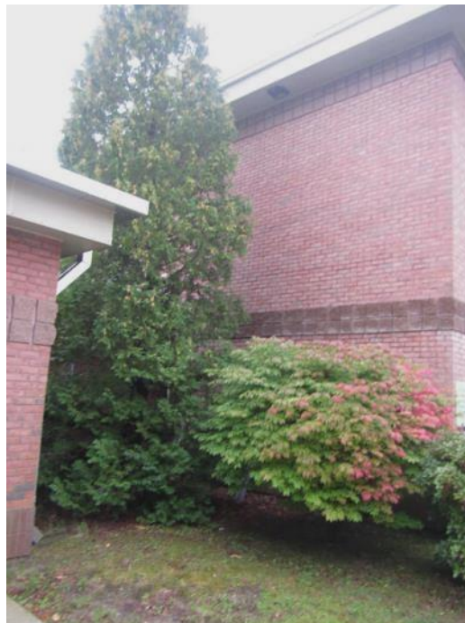
Trees/shrubbery in close contact with exterior walls
