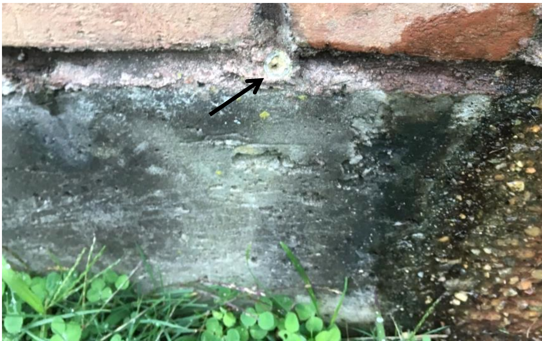
Clogged/plugged weep hole (arrow)
