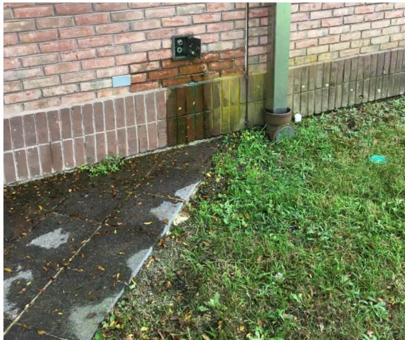
Leaking plumbing fixture
