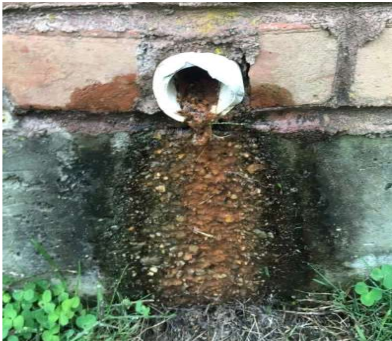
Debris/scale from condensate pipe/drip pans
