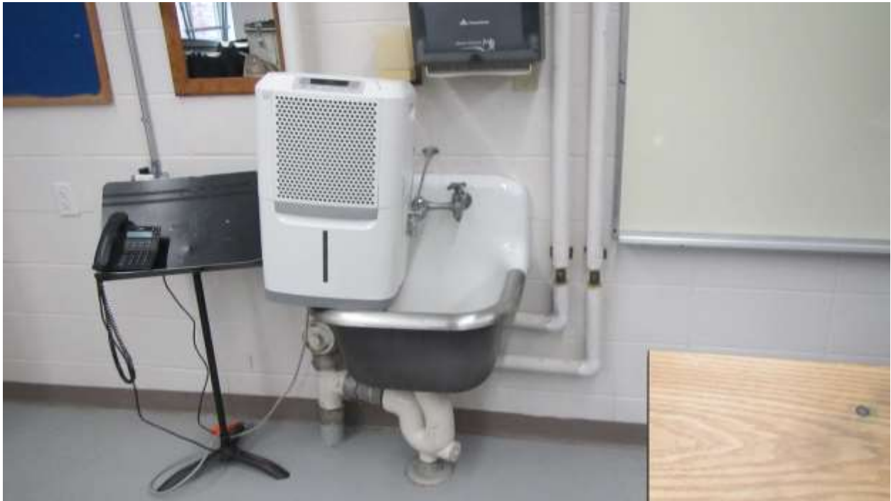
Custodial sink with mold odor from dry drain trap
