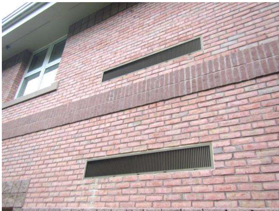
Univent fresh air intakes
