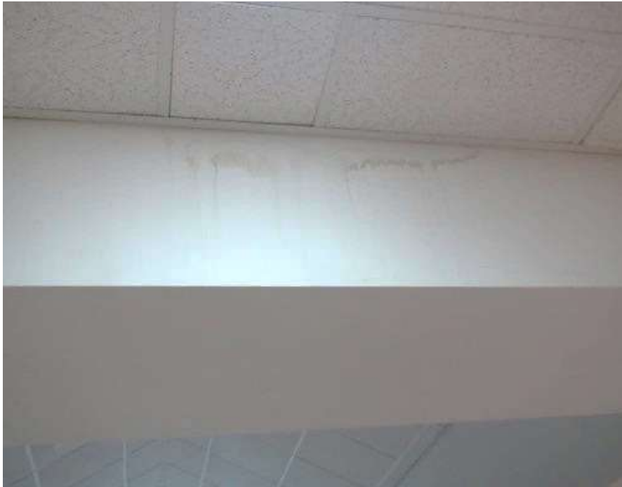
Water-stained gypsum wallboard outside Library
