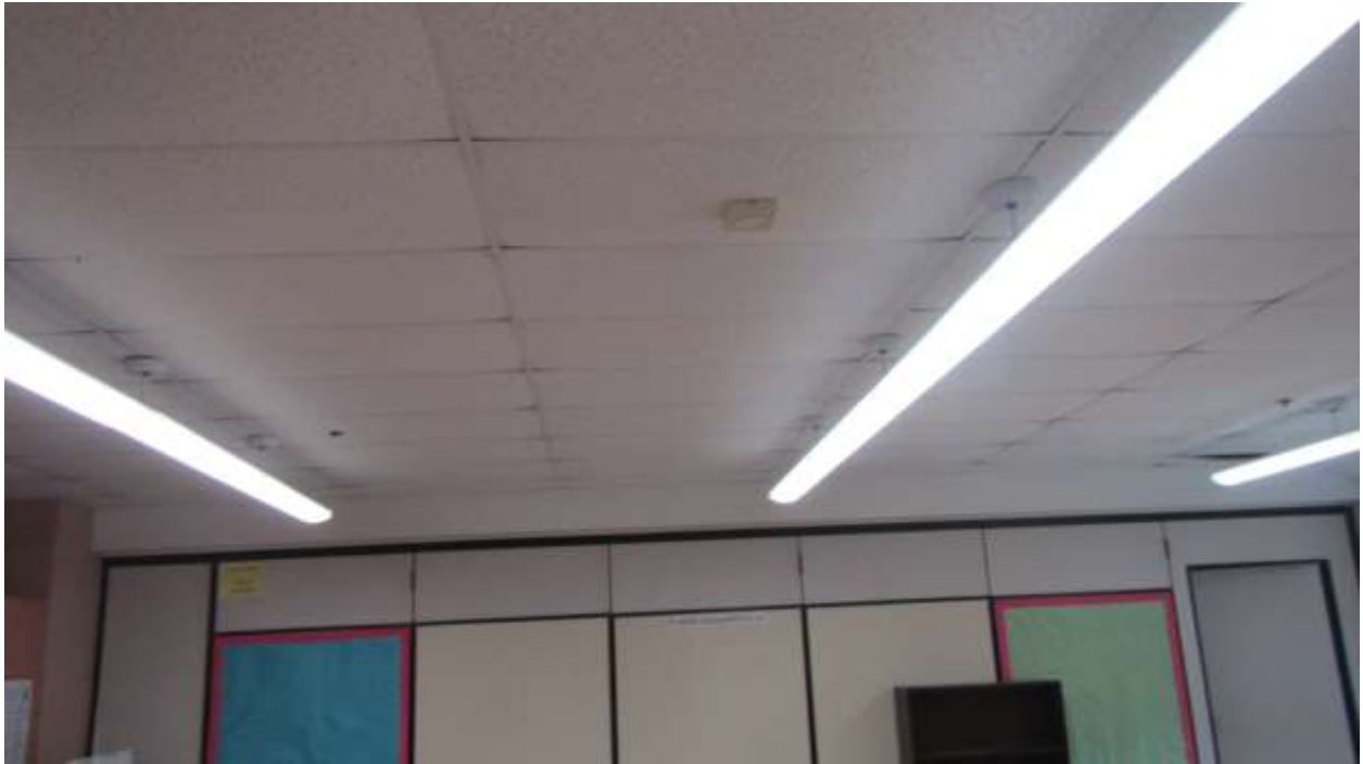
Bowed ceiling tiles
