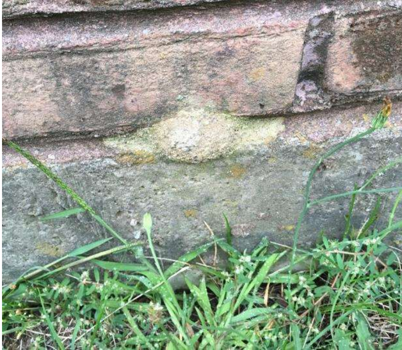
Clogged/plugged weep hole
