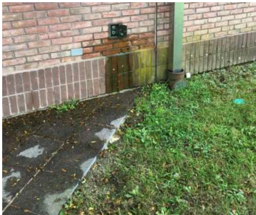
Leaking plumbing fixture
