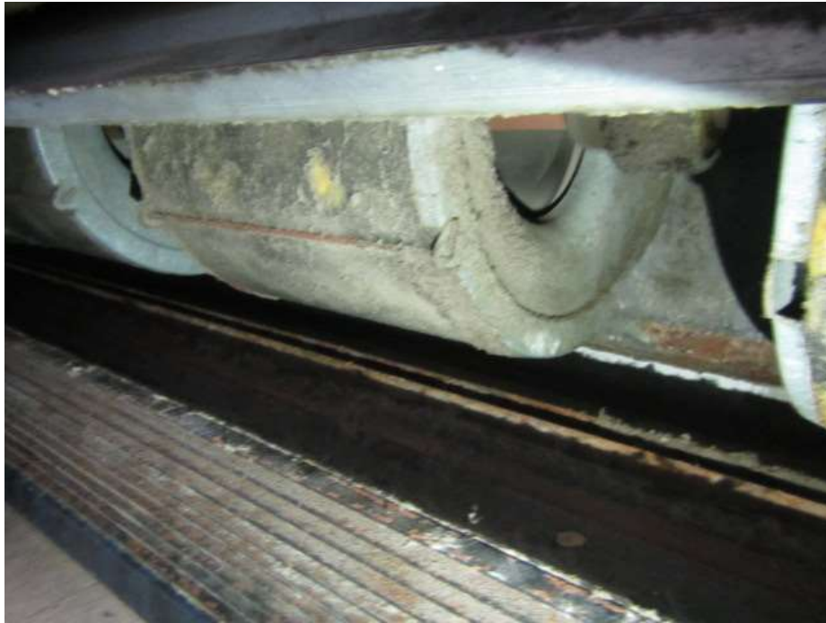
Accumulated dust/debris on interior univent components
