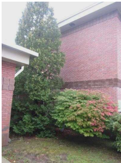
Trees/shrubbery in close contact with exterior walls
