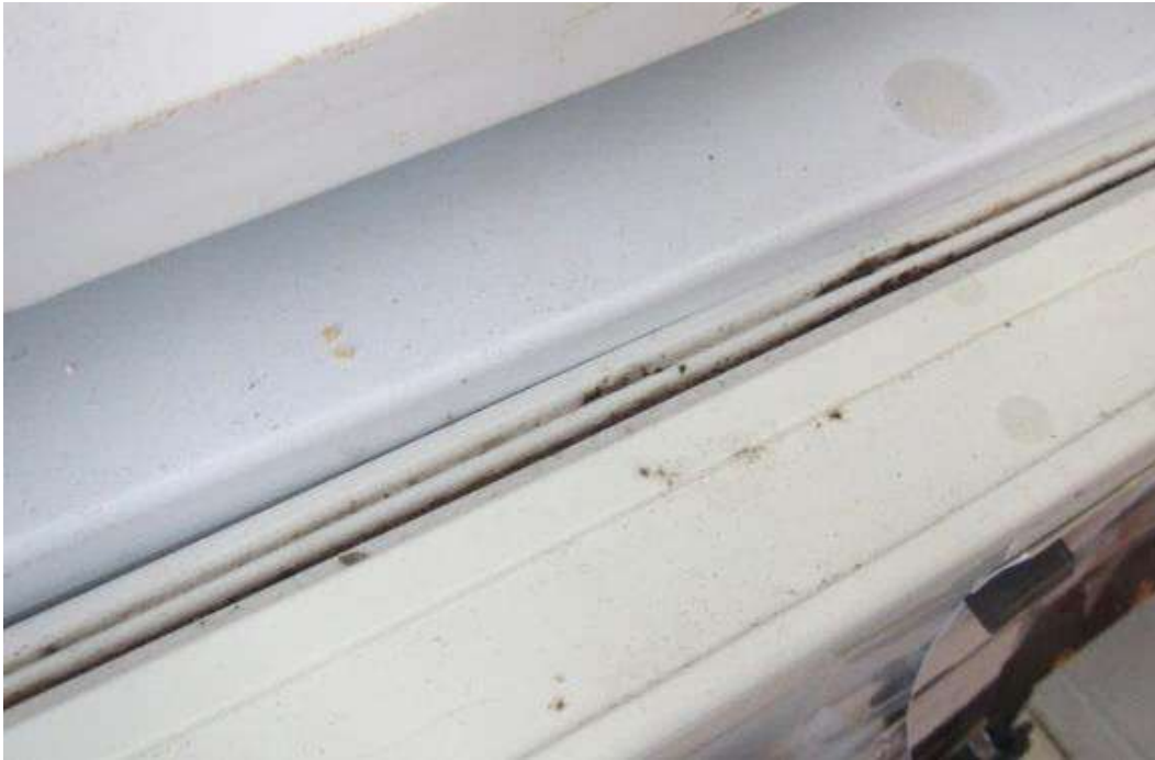
Debris/mold growth on mini-fridge gasket in classroom
