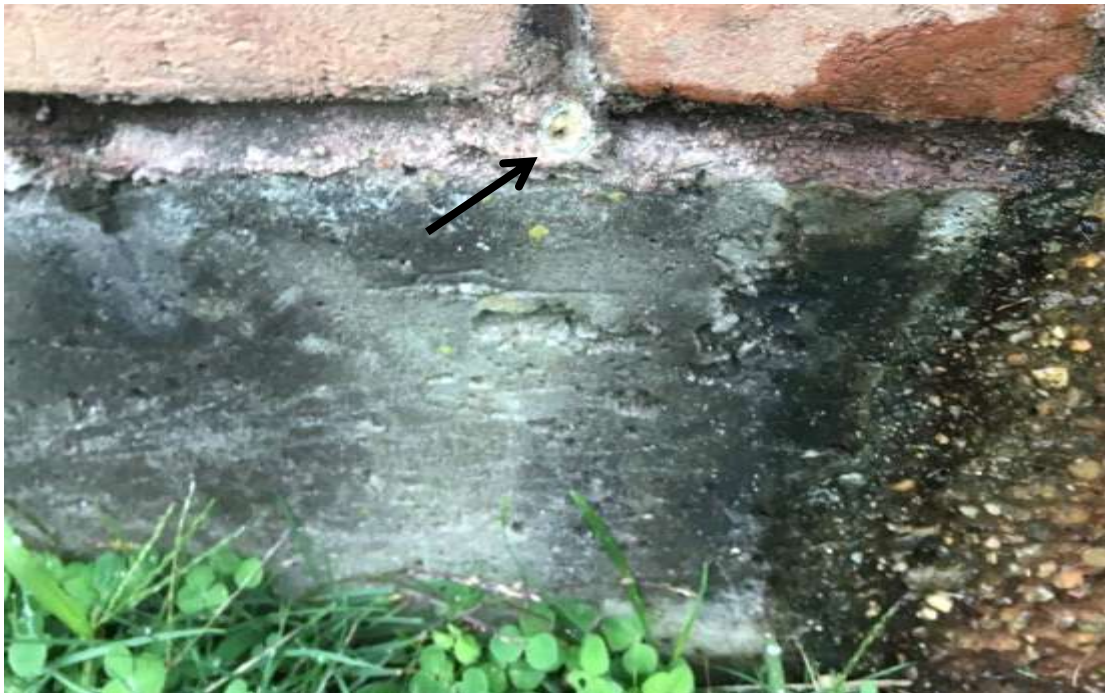
Clogged/plugged weep hole (arrow)
