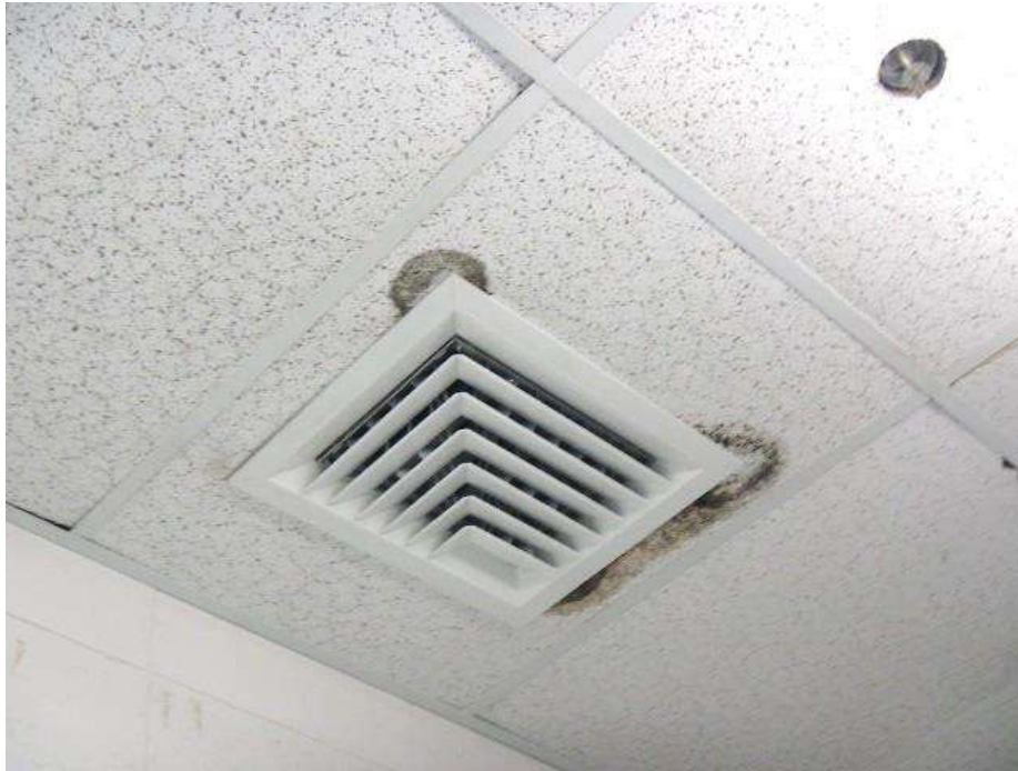
Water damage/mold growth on ceiling tiles room 107
