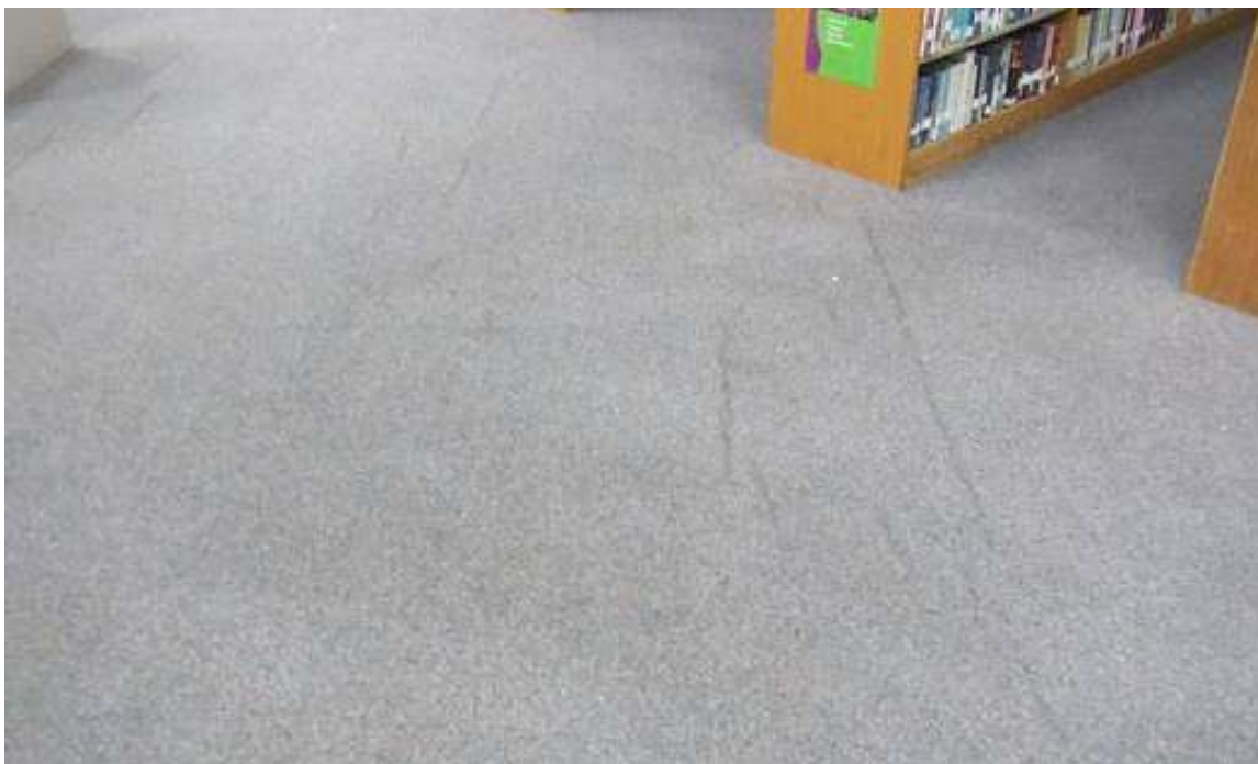
Original (20+ yr.)/wrinkled carpeting in Library
