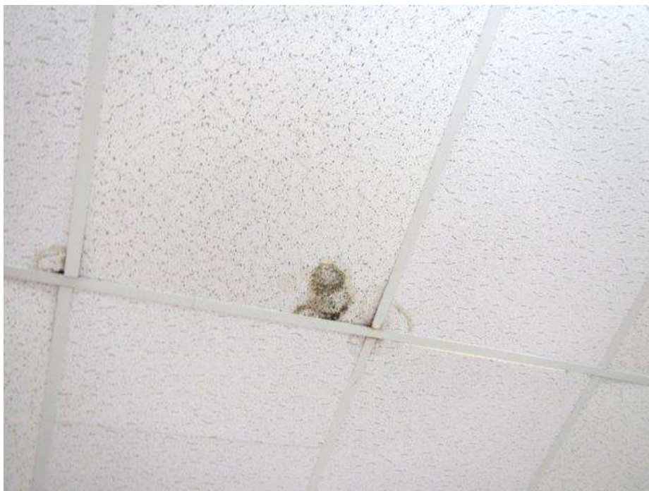
Water-damage/mold growth on ceiling tiles room 219
