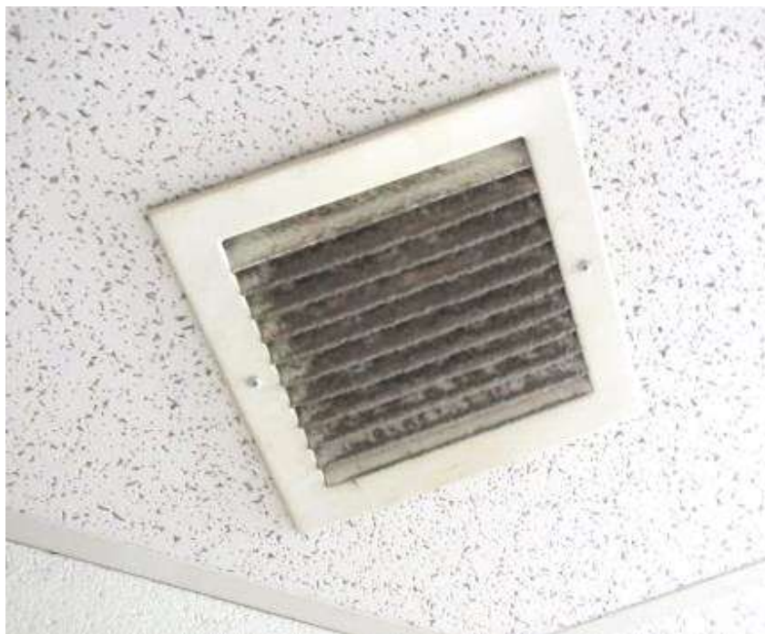
Classroom exhaust vent, note accumulated dust/debris
