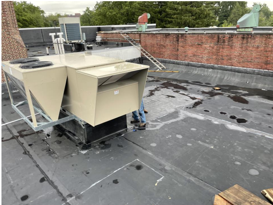
New RTU for Gym - Clinton Elementary School
