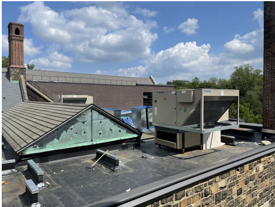
New Auditorium Roof Top Units - Jefferson Elementary School
