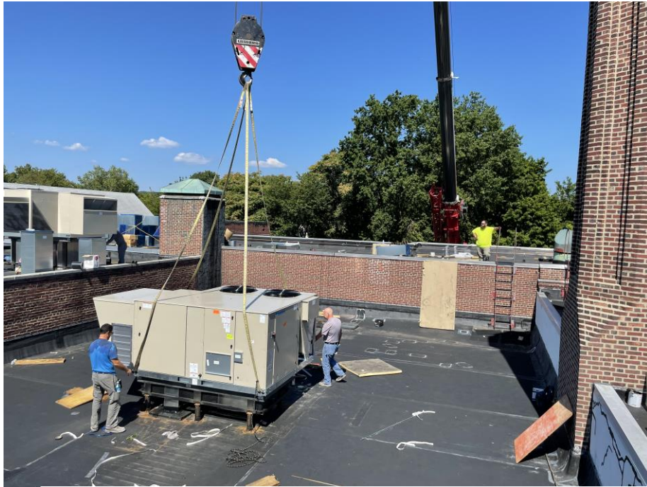
Gym New Roof Top Unit - Clinton Elementary School
