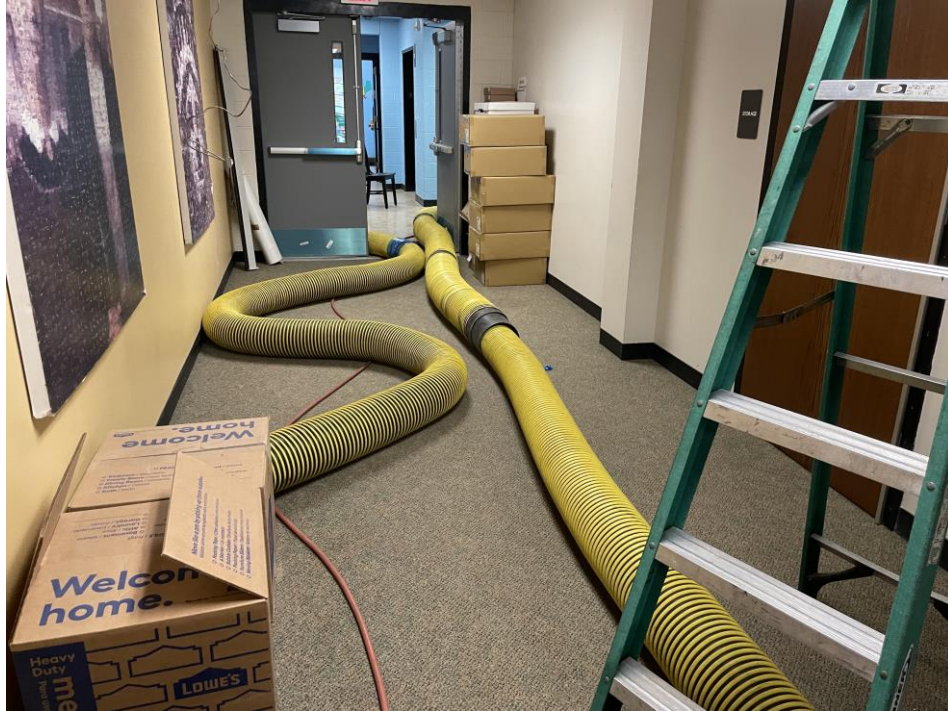
Existing Ductwork clean out at Media Center - Jefferson Elementary School
