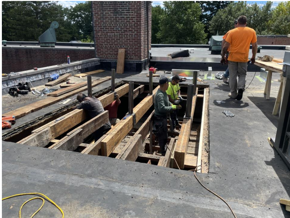
Added Structural Supports at existing Auditorium roof for new RTU's - Clinton Elementary School
