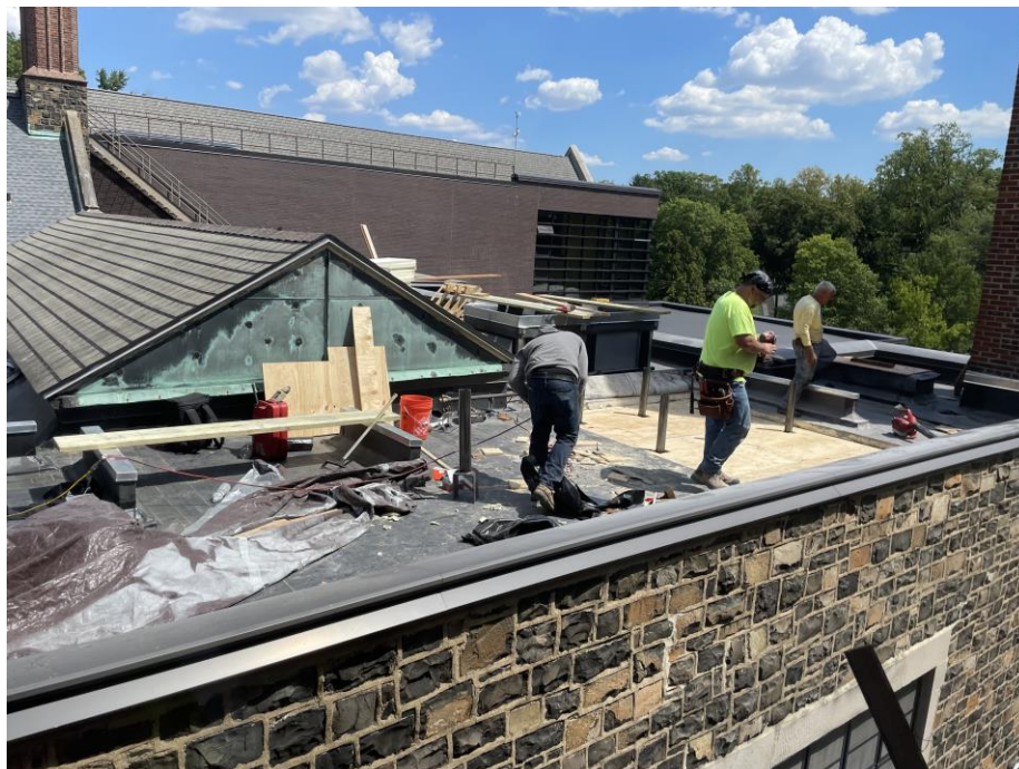
Steel supports for new RTU's - Jefferson Elementary School
