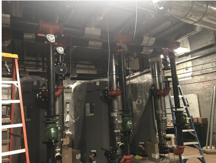
New Boilers and Breeching - Jefferson Elementary School
