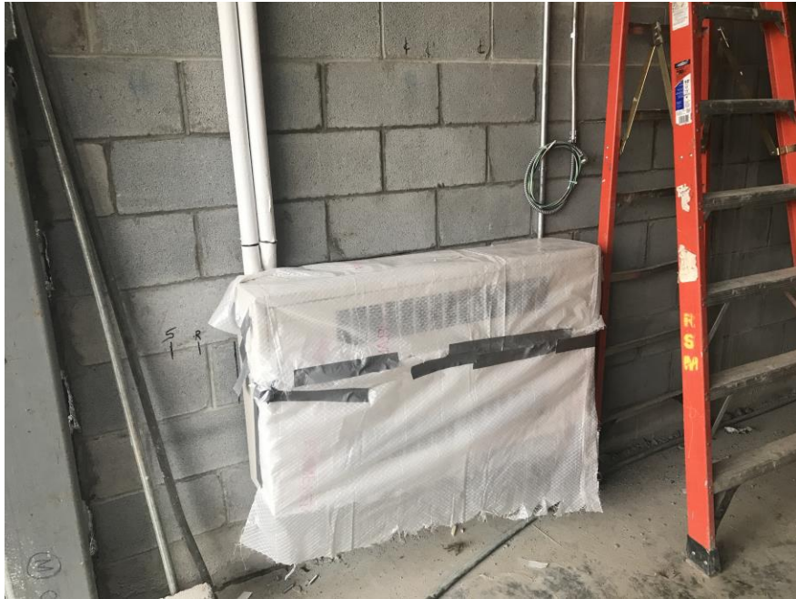
New Cabinet Heater at entrance - Clinton Elementary School
