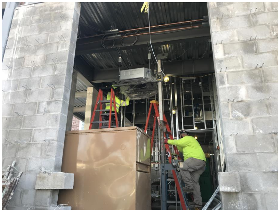
Mounting Units in office at area A - Clinton Elementary School
