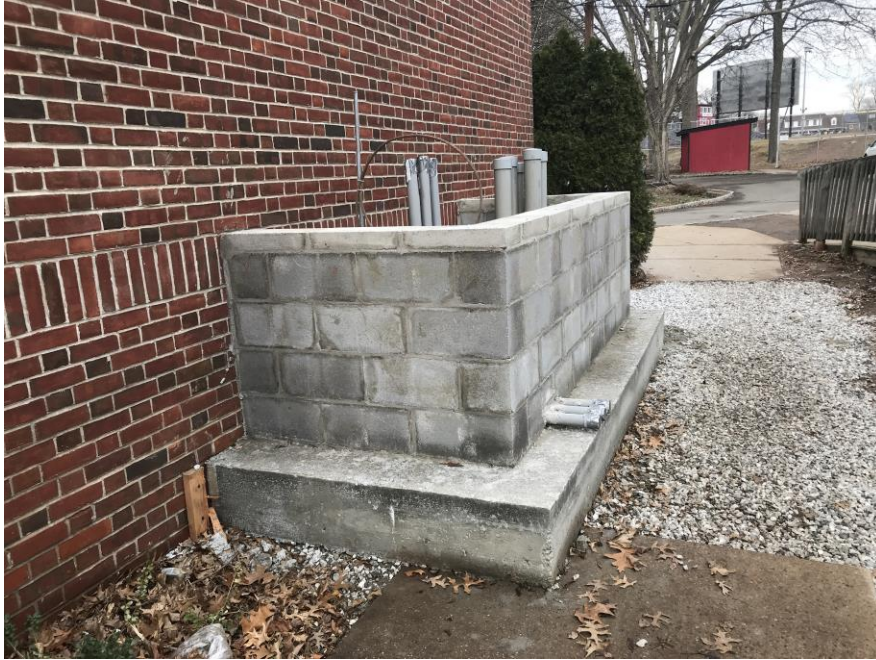
CMU Block at Switchgear - Clinton Elementary School
