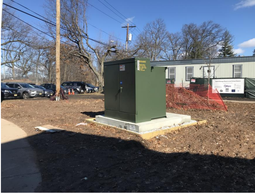
New Transformer - Clinton Elementary School
