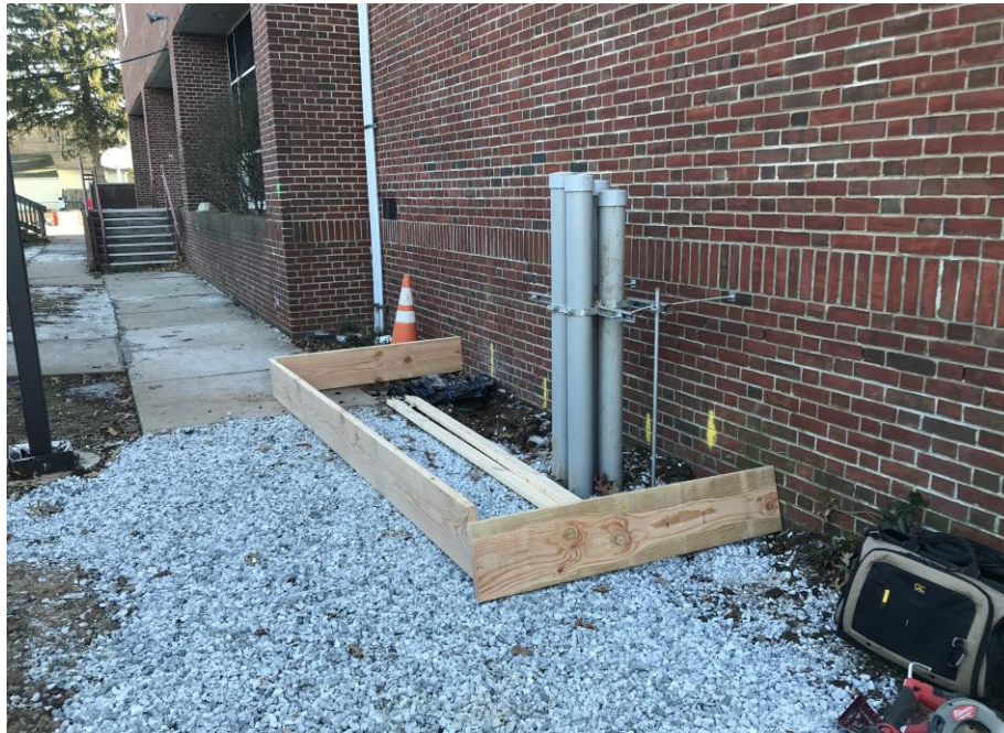
Box out for new slab at New Switchgear location - Clinton Elementary School
