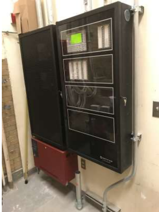
New Fire Alarm Panel (Activated)– Clinton Elementary School
