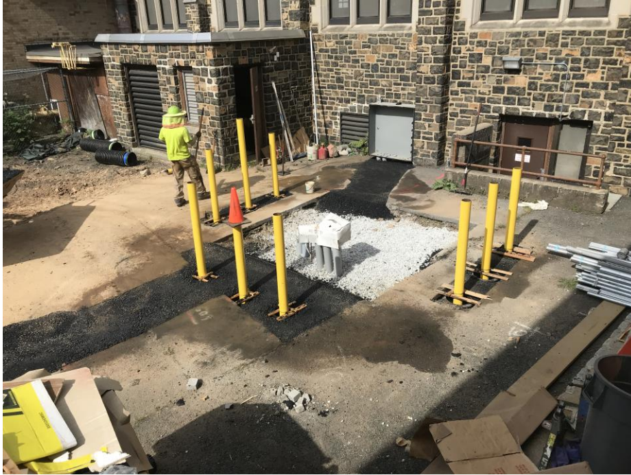
New Transformer location– Jefferson Elementary School
