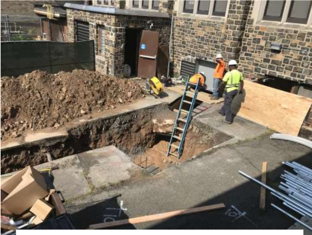
Trench and transformer Pad located – Jefferson Elementary School
