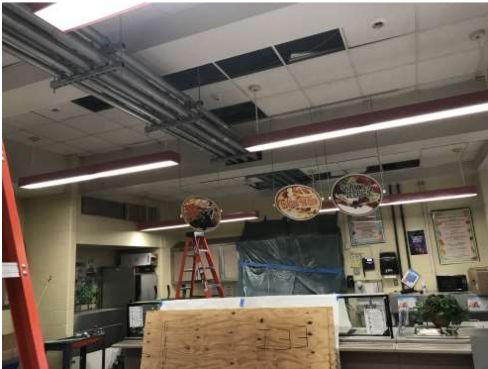
New Feeder mains– Clinton Elementary School
