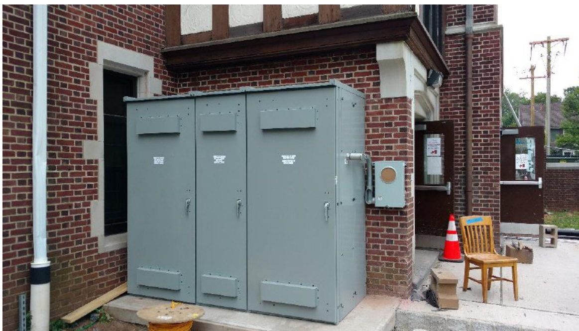
Tuscan School- Exterior Switchgear
