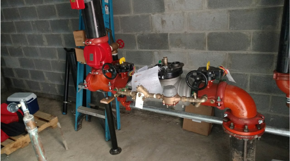
Seth Boyden School- Sprinkler System Back-flow/Check Valve
