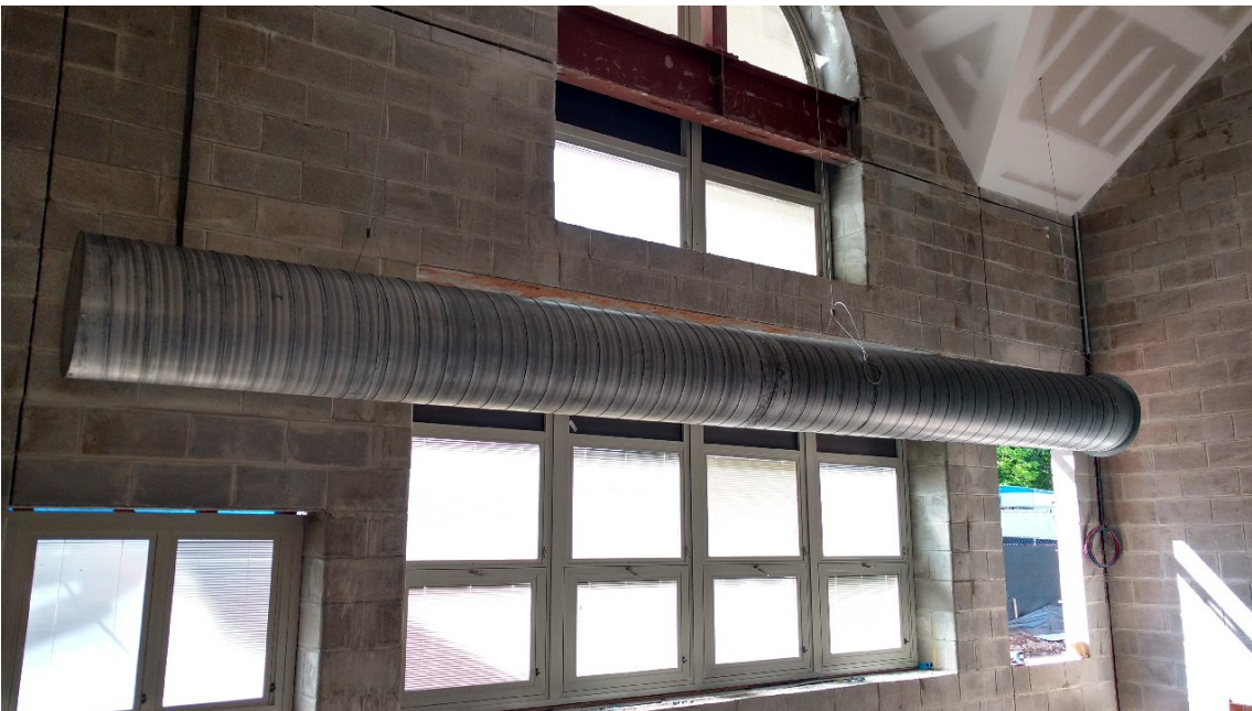
Tuscan School - Classroom Ductwork
