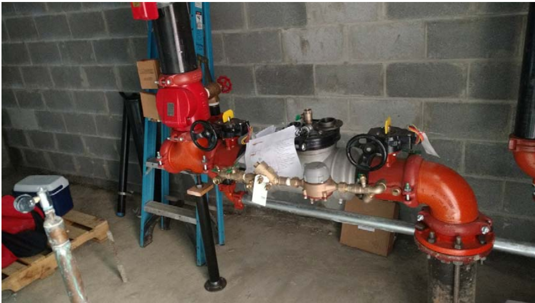
Seth Boyden School - Sprinkler back-flow and check valve assembly
