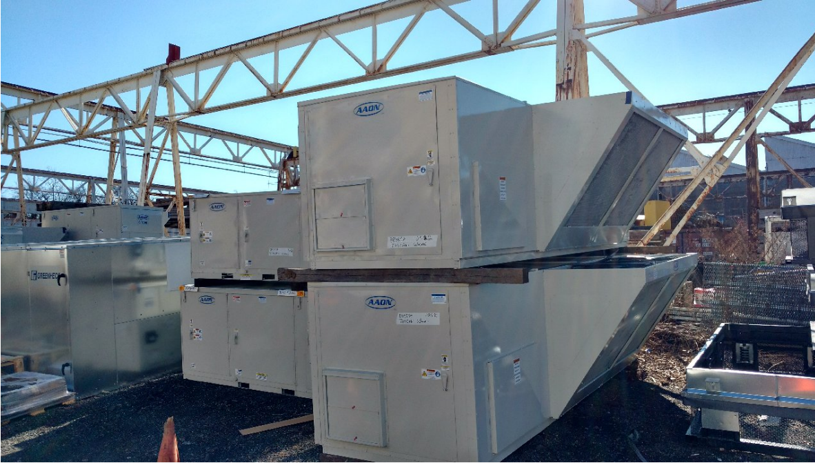
Tuscan School - HVAC Units in Storage Yard
