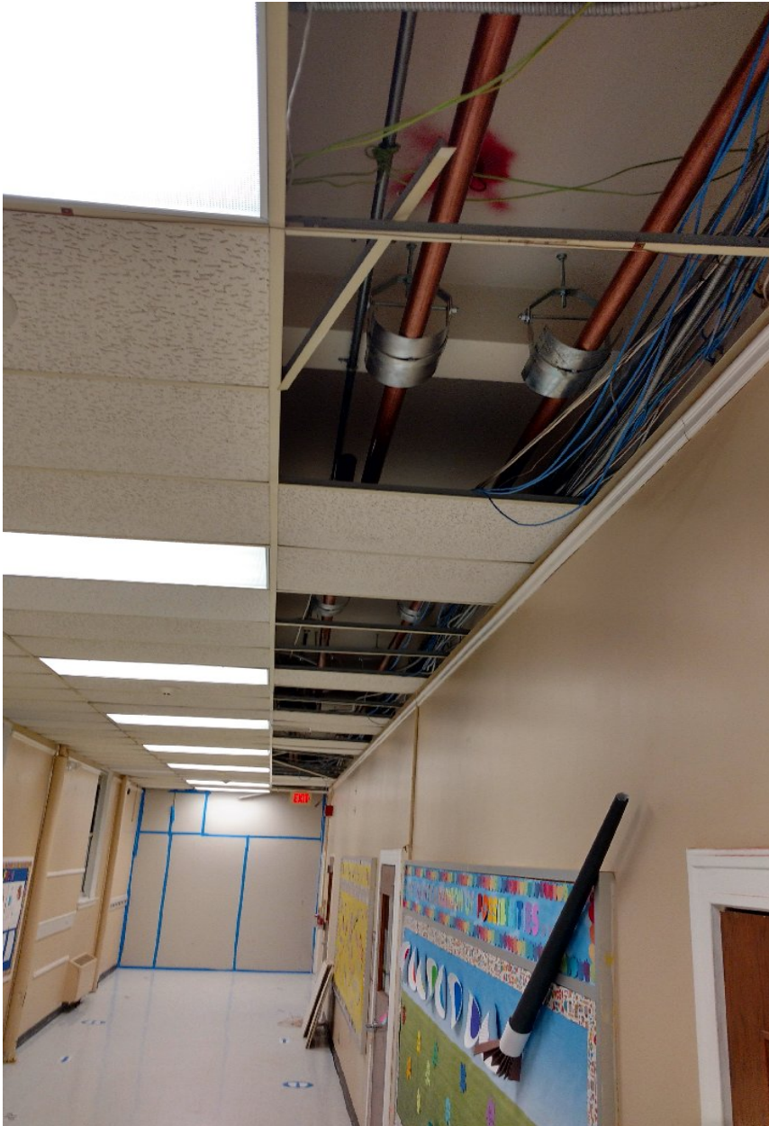
Seth Boyden- Hydronic Piping at the ceiling
