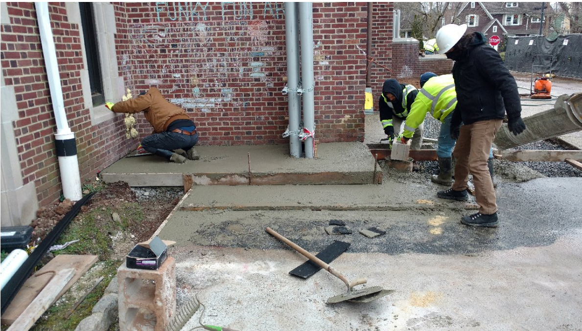
Tuscan School - New Electrical Switchgear Pad
