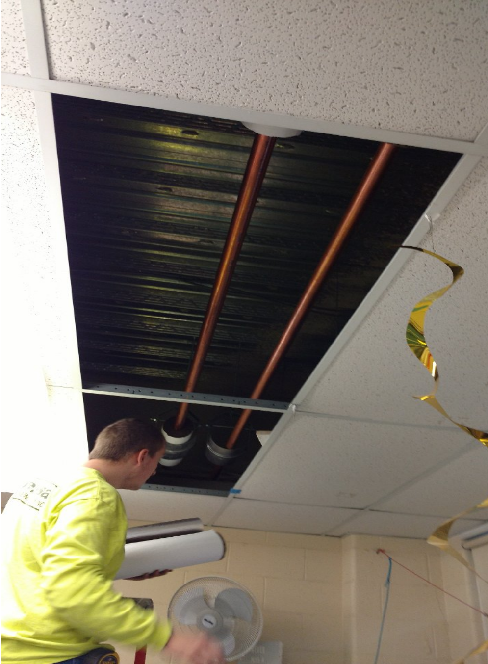
Seth Boyden - Hydronic Piping Insulation at the classroom.
