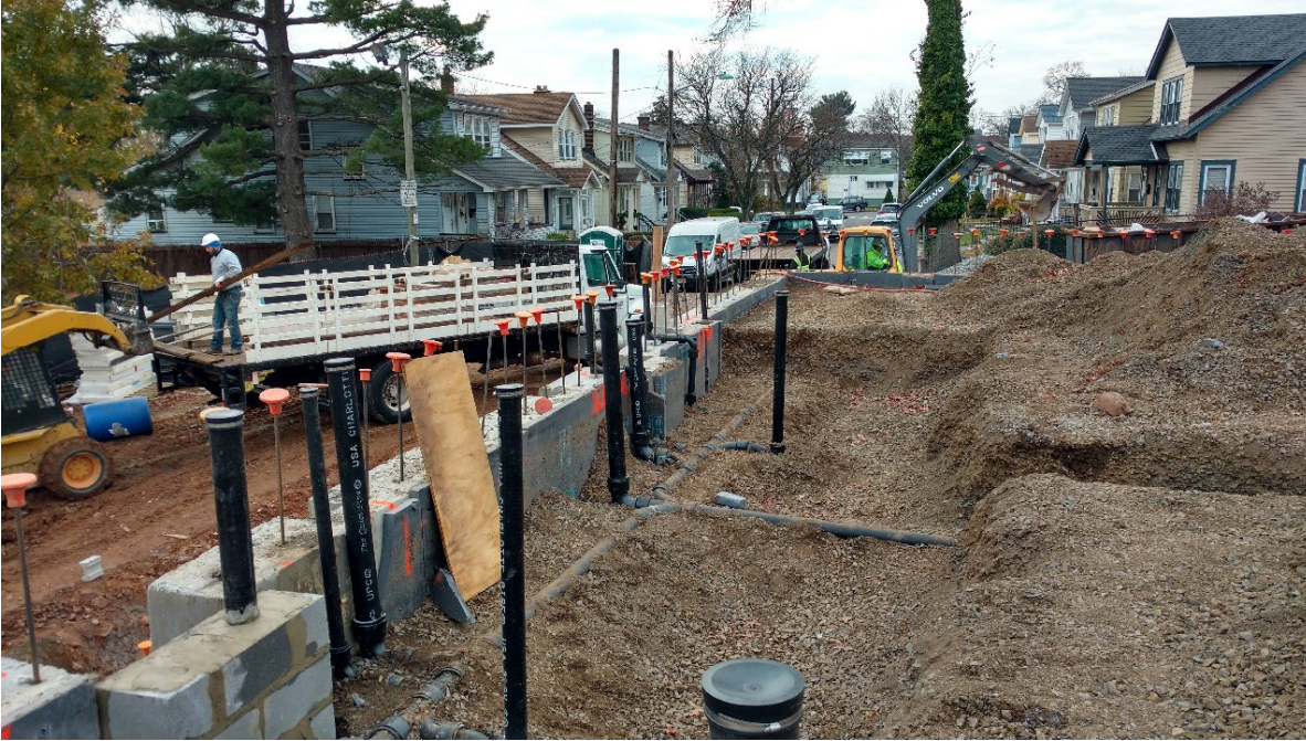
Seth Boyden- Underground sanitary piping's
