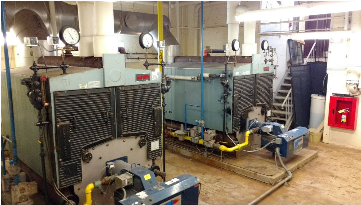
Tuscan School - Two Existing boilers to be removed
