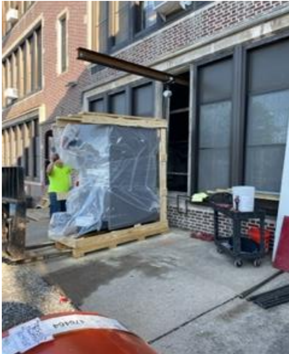
New boilers at SME
