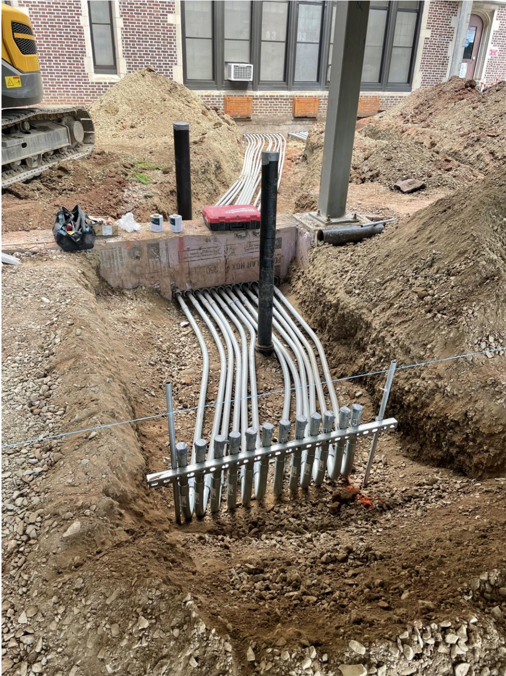
Underground electrical conduit at SME
