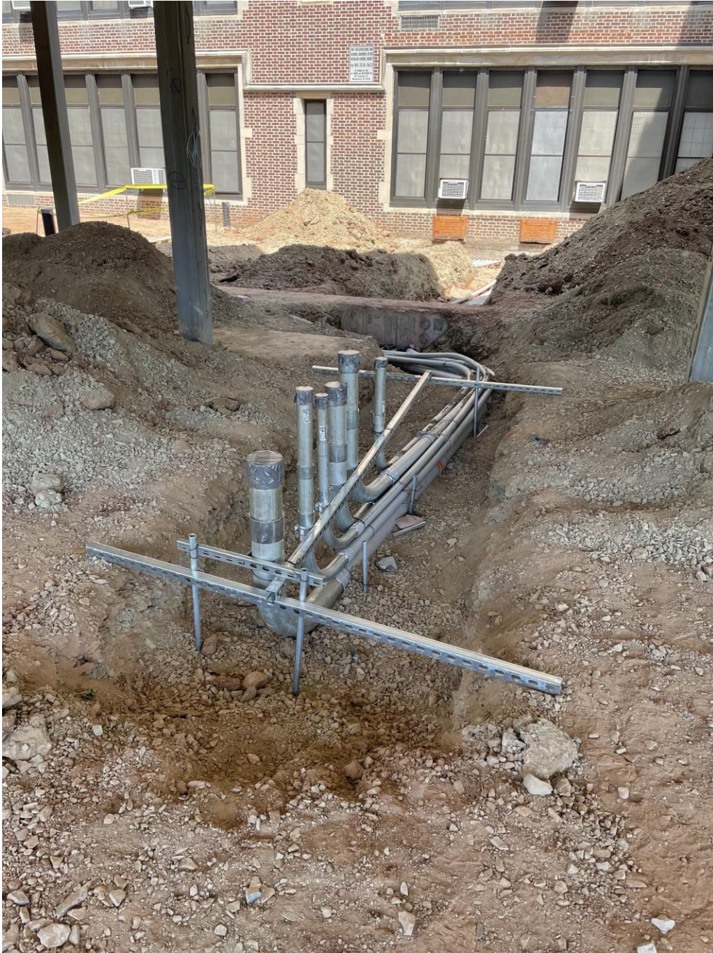
Underground electrical conduit at SME
