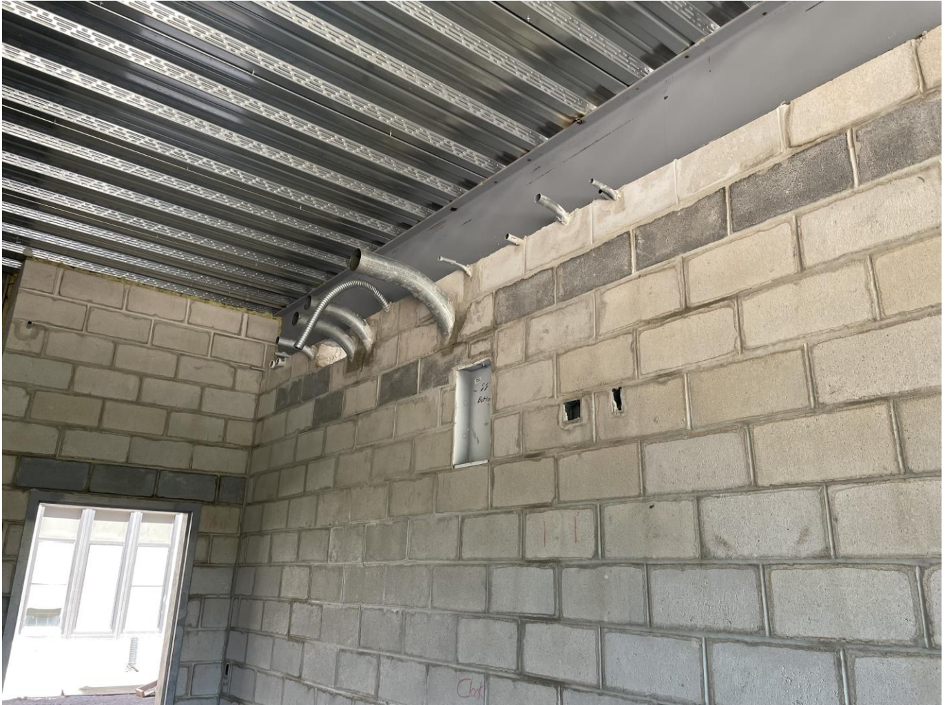
In-wall electrical conduits and back boxes at SME
