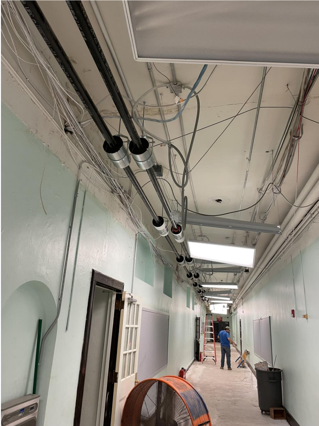
HVAC supply & return piping at SME
