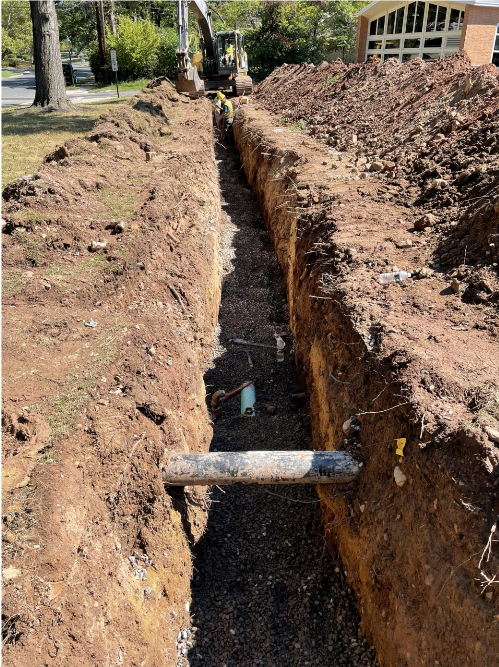
Sanitary sewer at SMA
