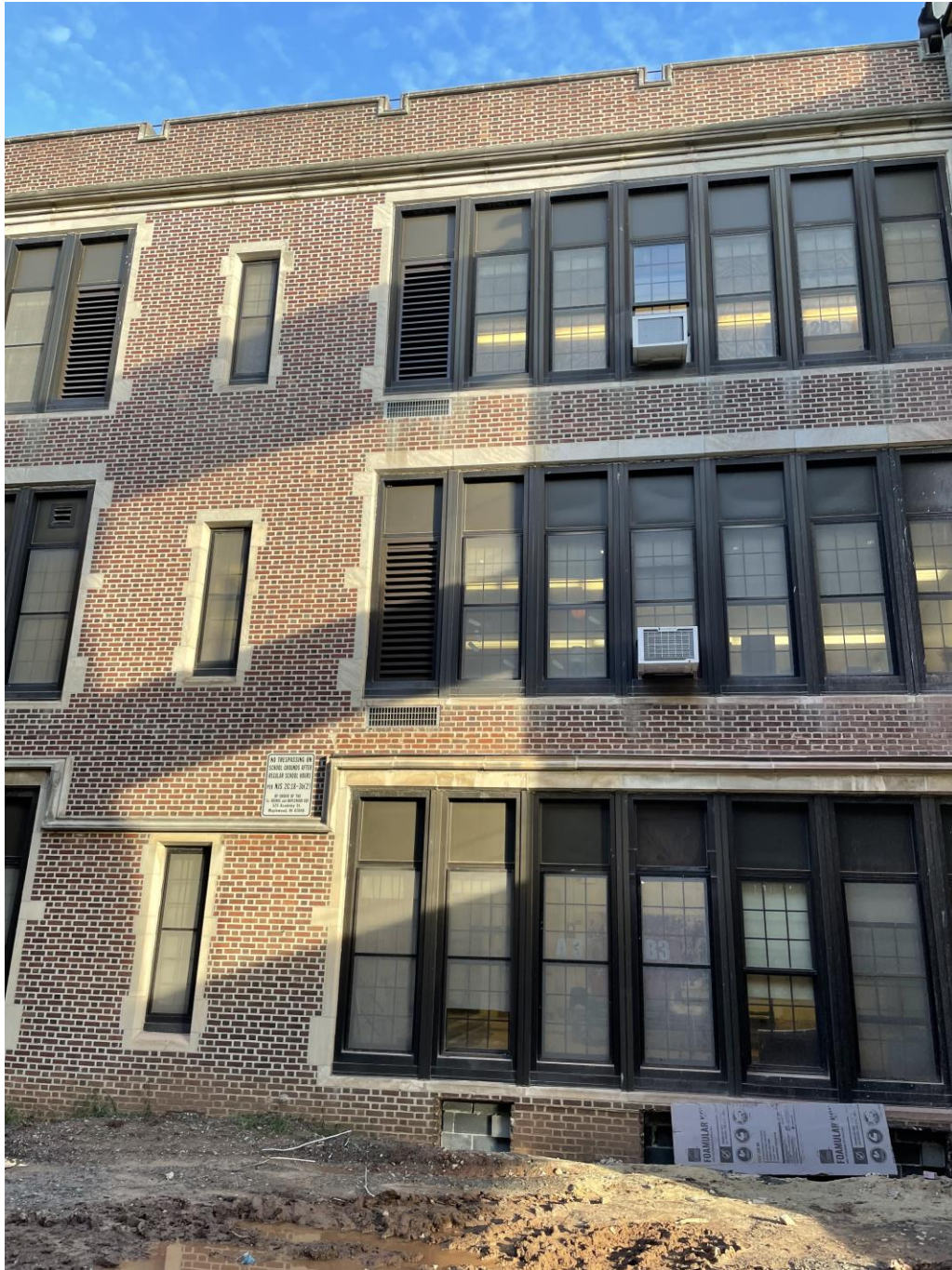
VUV louvers installed at SME
