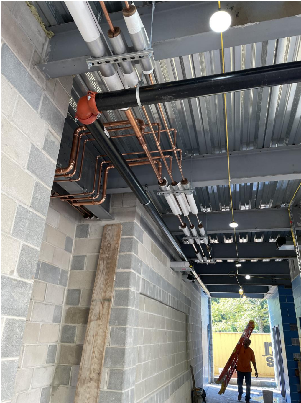
Fire sprinkler piping at SME
