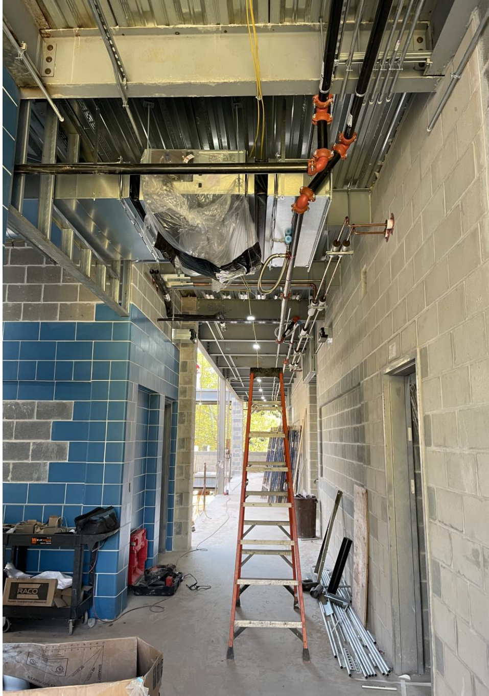
VRF Evaporator units, sprinkler and plumbing at SME
