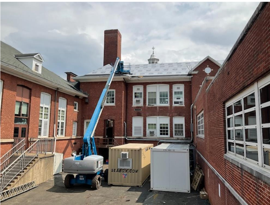
Area B facing Dunnell Road Slate Roof Replacement with Asphalt Shingles- continues. (Roofing 80% or more completed)
