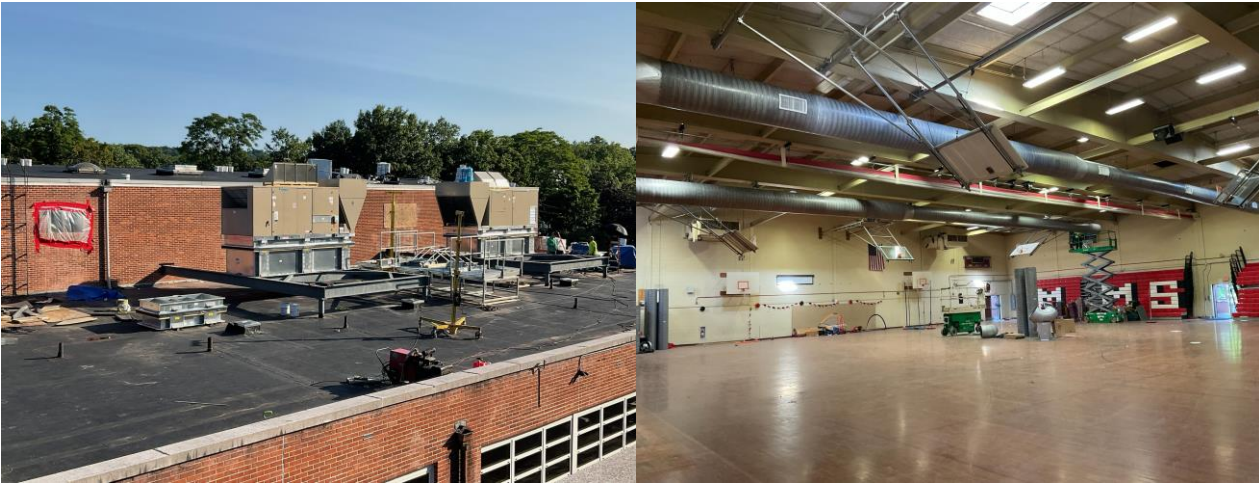
Left- Gym AC Units Lifted into place. Right- Gym ductwork underway. Demo of legacy AHUs started.
