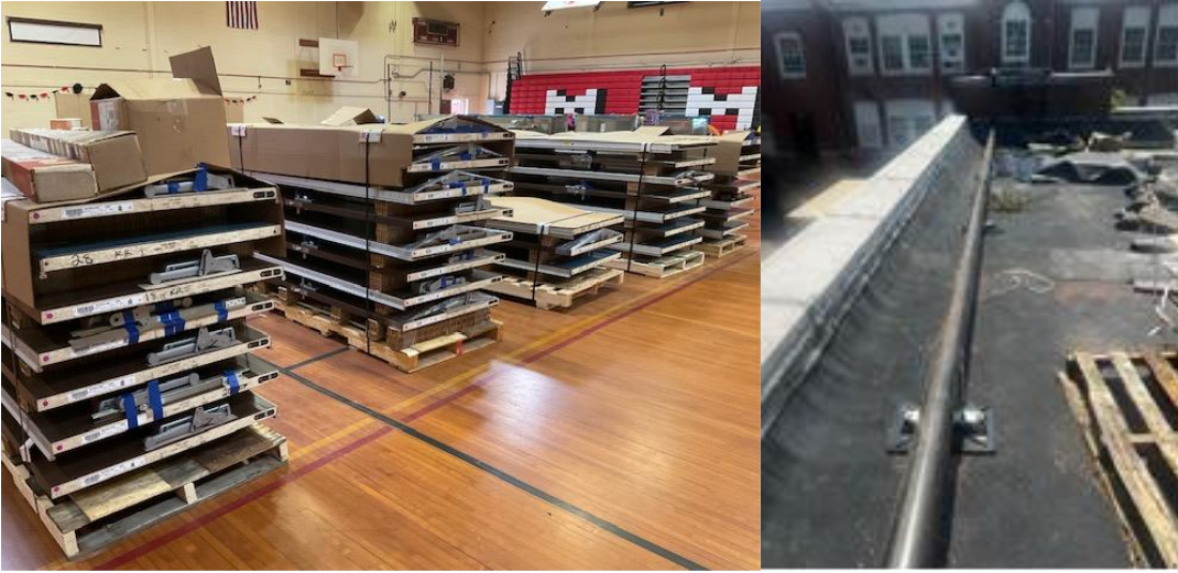
Gym- Left: New interior room doors staged. Right: New gas line serving rooftop units.
