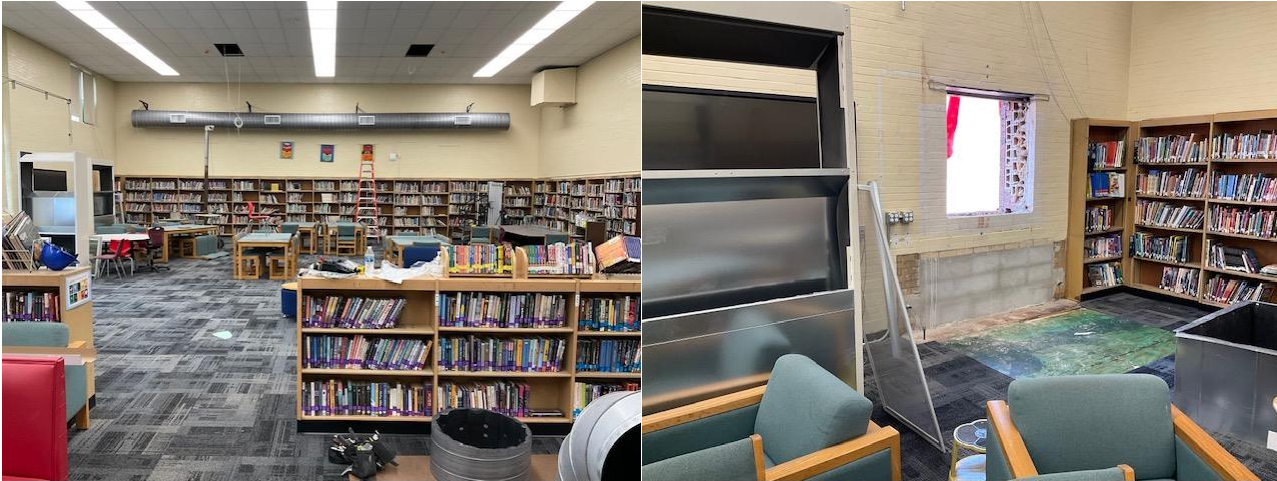
Library: Left: Ductwork trunks installed (one shown). Right: VUV louver opening created.
