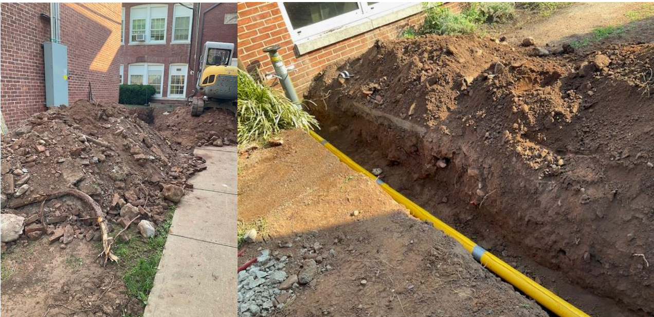
Exterior Trenching- Left: Electric for back feed of existing loads & Right: Gas pipe for rooftop units.
