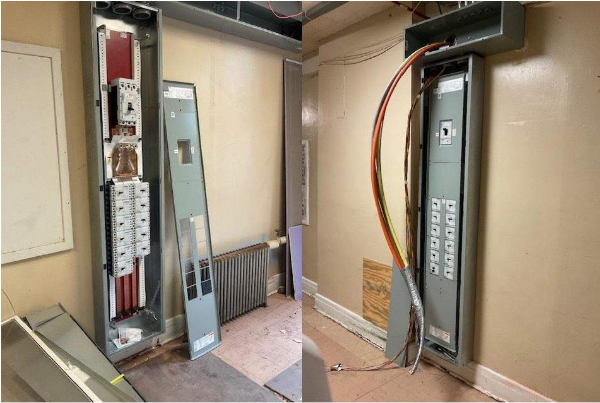
VUV Electrical Panels in Corridors- breakers installed, wires pulled. 5 Panels in total.
