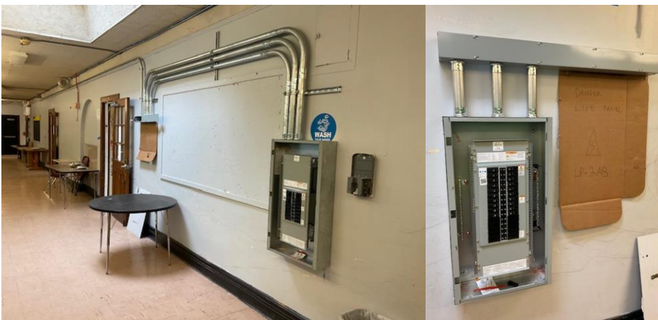
New Lighting Panels throughout interior
