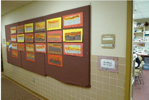
Delaminating tackable surface
