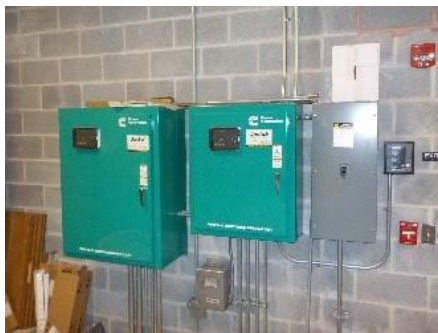
Emergency transfer switches
