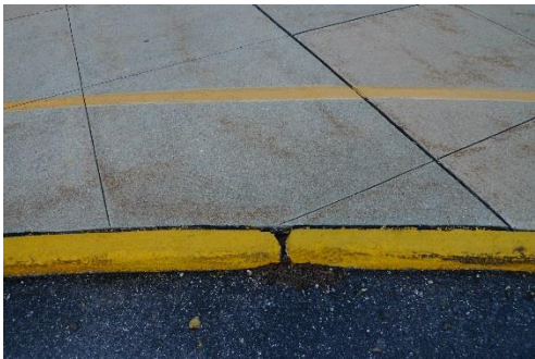
Portion of deteriorating curb at main entrance
