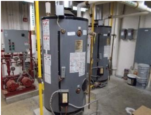
Domestic water heaters
