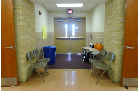
Egress path obstructions
