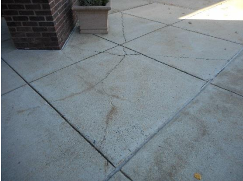
Area of heave and drop with cracking
