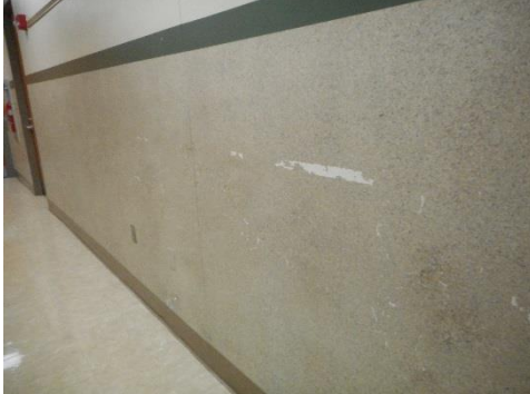
Damaged GWB with specialty paint
