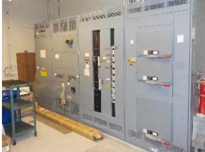
Main electrical switchgear
