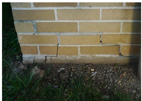
Typical brick and mortar deterioration
