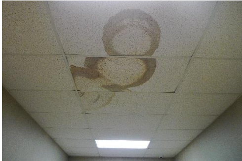
Visible water damage at ACT ceiling
