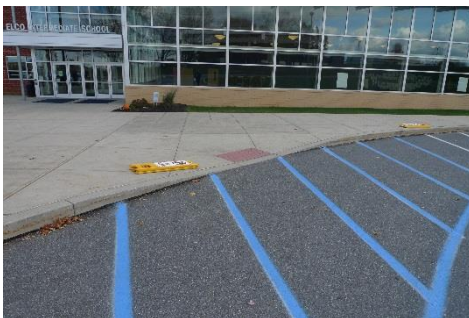
Curb at building entrances
