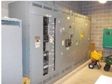
Main electrical switchgear
