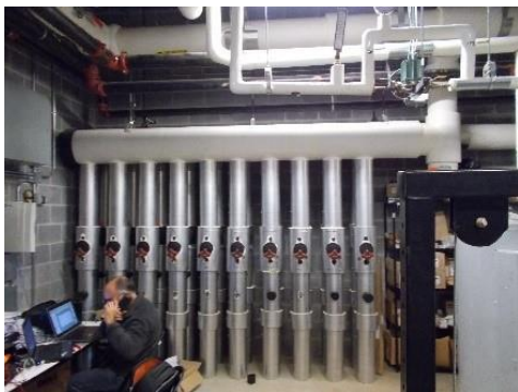
Geothermal manifold piping
