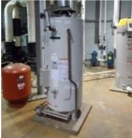
Kitchen domestic water heater
