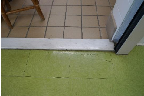
Transition at cafeteria to kitchen – trip hazard
