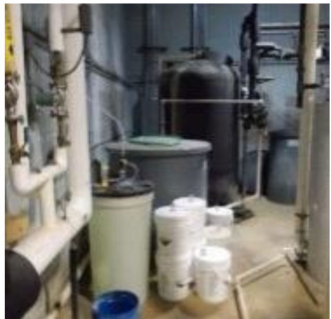
Water softening system
