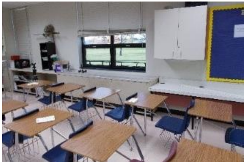
Typical classroom unit ventilator
