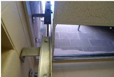
ACT at roof access
