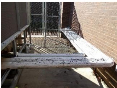
Exterior piping insulation
