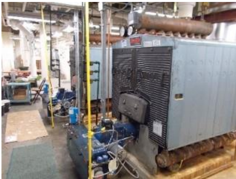
Hot water boilers
