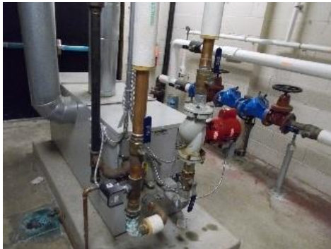
Domestic water heater
