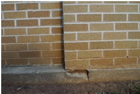
Concrete deterioration at base
