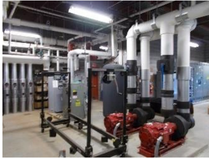
Domestic water heaters
