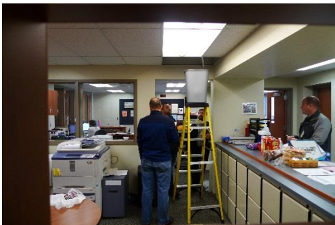
Water containment at the front office
