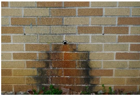
Typical water discharge and deterioration
