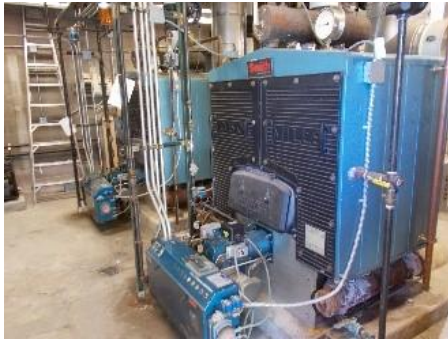
Hot water boilers
