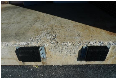
Deteriorating concrete loading dock edge
