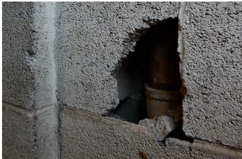
Deteriorated block at interior
