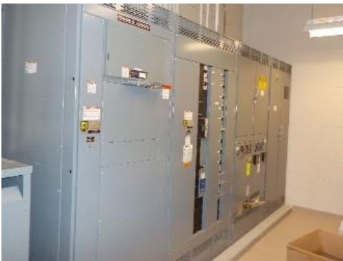
Main electrical switchgear
