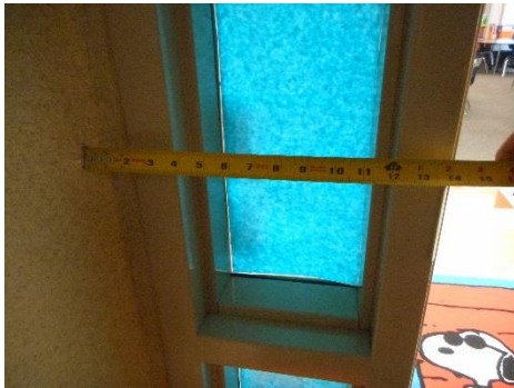
Pull side access width does not meet code
