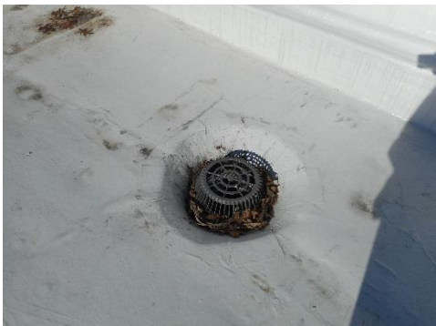
Roof drain with debris
