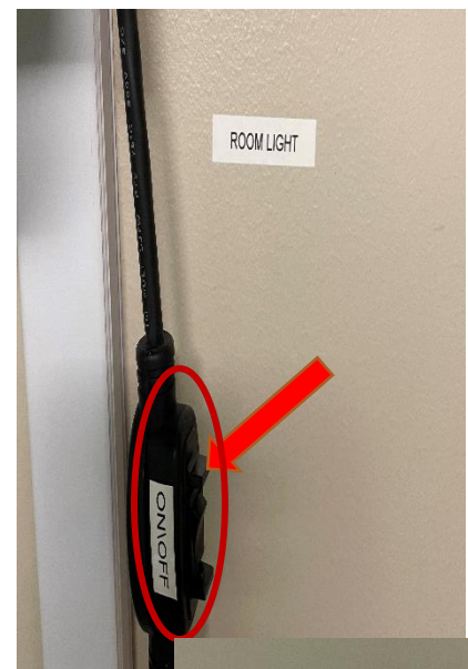
Room Lighting – on/off
