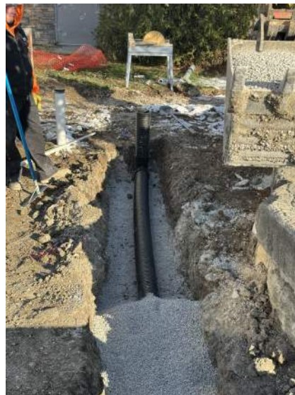
PR04 Storm Drains
