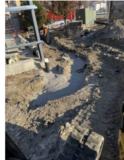
PR04 Storm Drains
