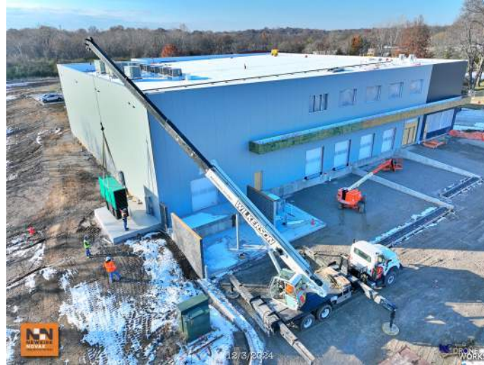
East Lot/Generator Set
