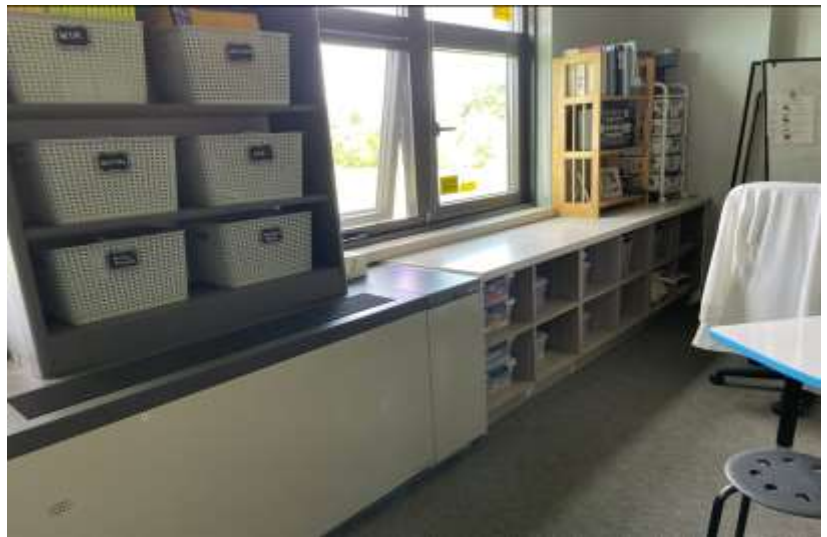
WBS - Classroom new HVAC unit + adjacent shelving
