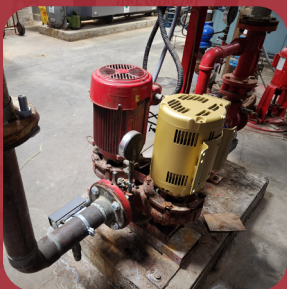
Water Pump System
