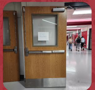
Broken Door Repairs
