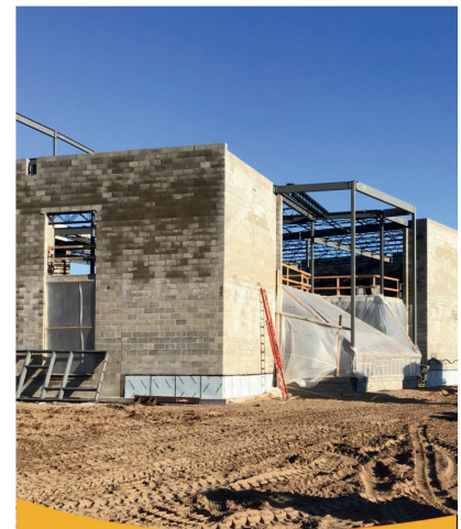
Walls are up on classrooms at the new elementary school. Who's classroom will this be?
