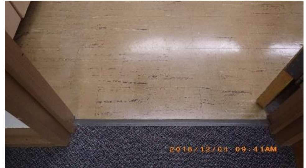
Vinyl Asbestos Tile
