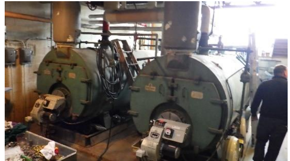
Heating Water Boilers
