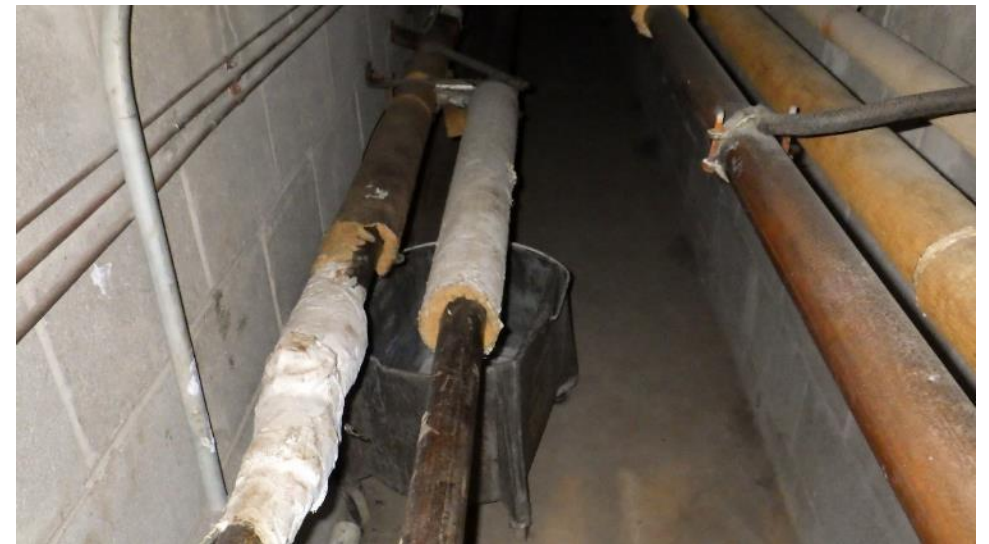
Piping in tunnel with missing insulation
