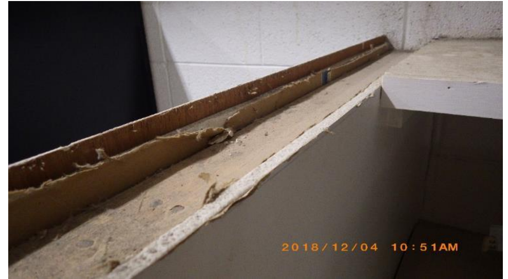
Wood Framed Walls Not Allowed
