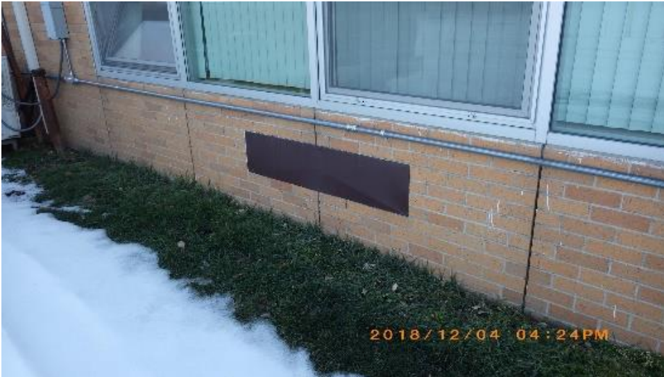
Classroom Ventilation Air Opening Covered
