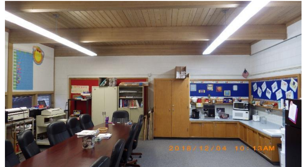
Lighting – Suspended T8 fluorescents
