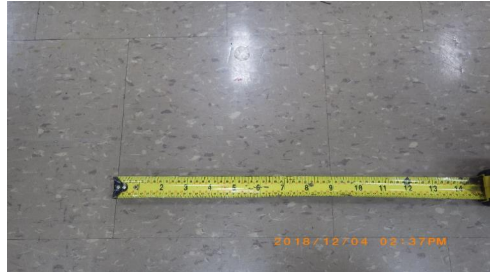
Vinyl Asbestos Tile
