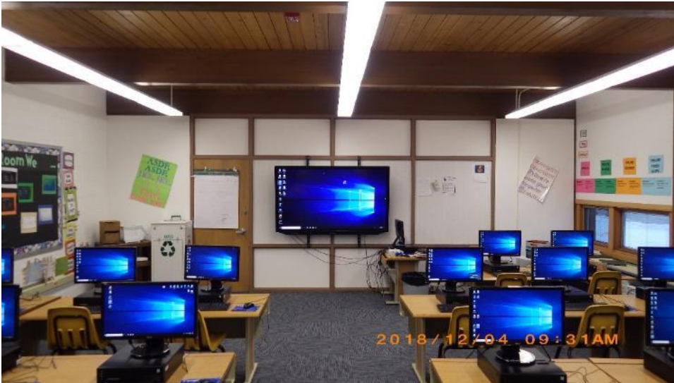
No Fire Suppression System
