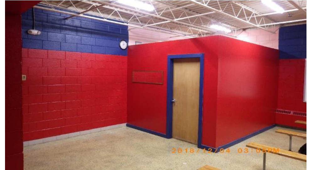
Wood Framed Walls Not Allowed
