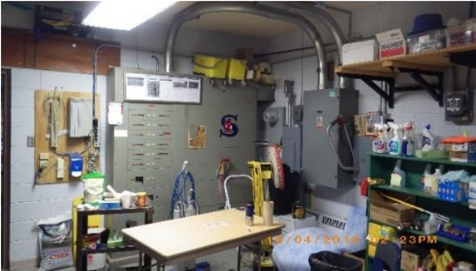
Electrical Service (mostly original)
