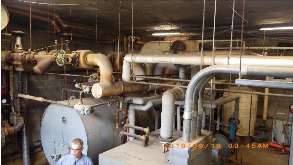
Pipe Insulation / Elbows
