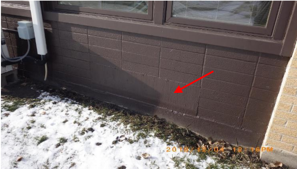
Classroom Ventilation Air Opening Covered
