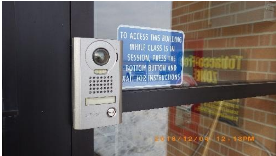
Signage & video-intercom at main entry
