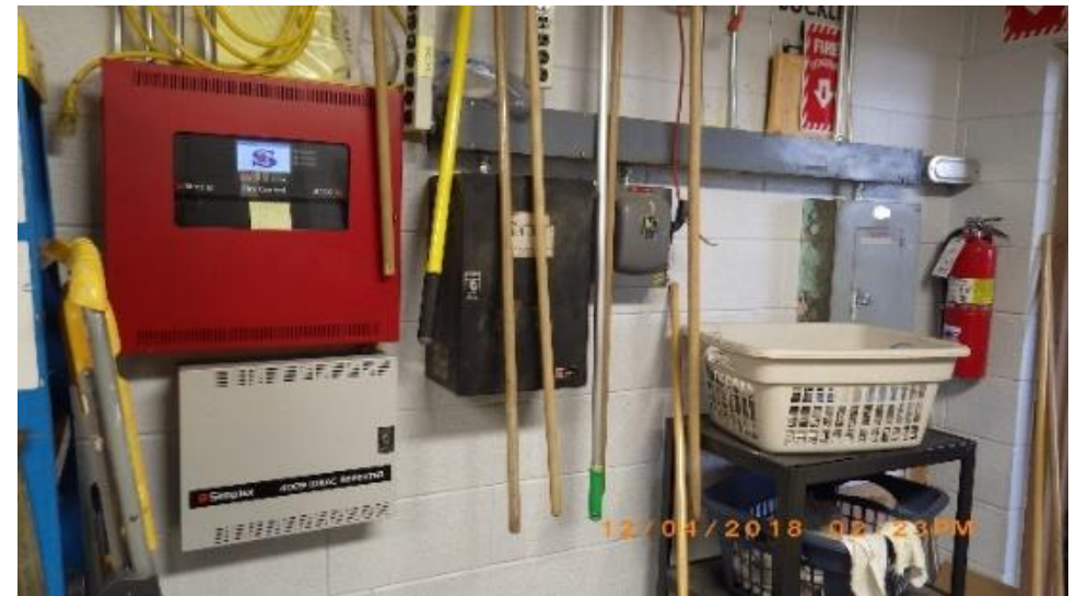
Fire Alarm (new, but obsolete)
