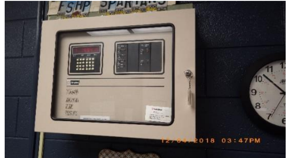
Master Clock (issues, being replaced)
