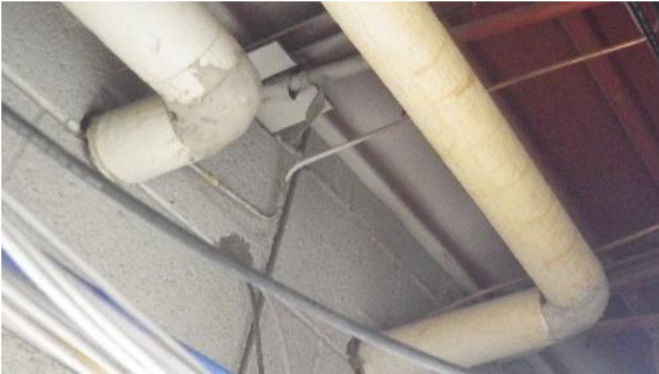
Pipe Insulation / Elbows
