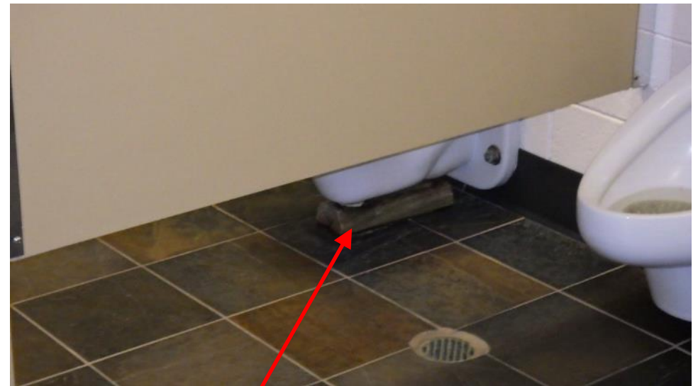
Wood blocking supporting toilet.
