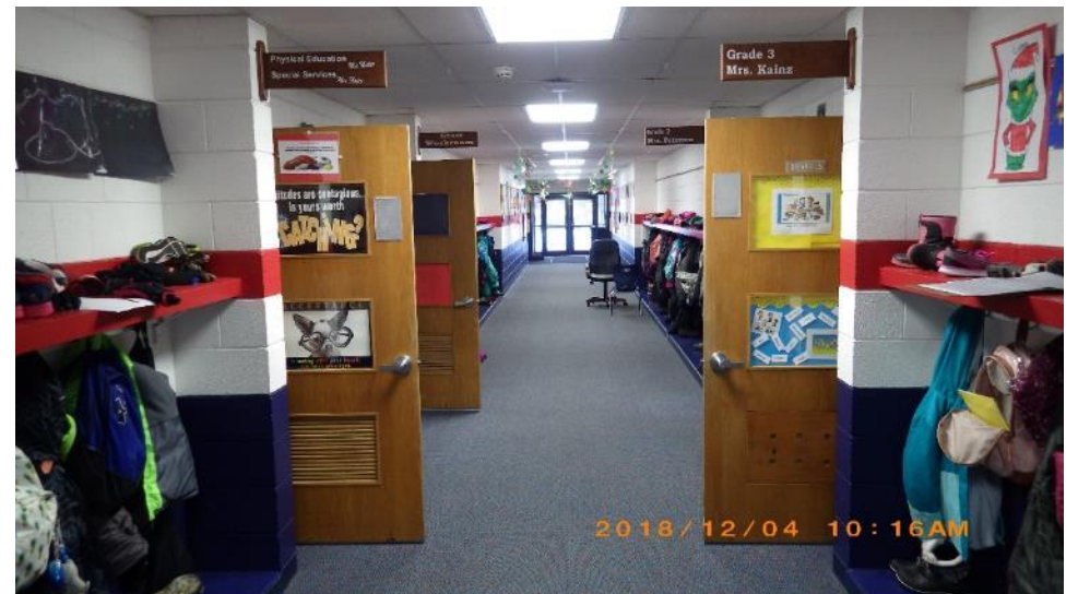
Restricted Corridor Width / Combustibles (No lockers)
