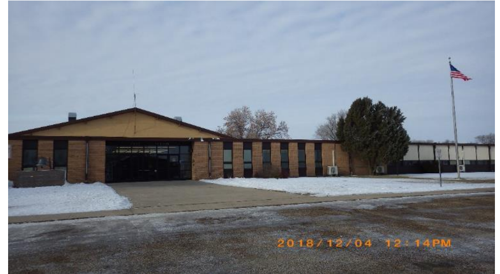
Lack of ADA Parking
