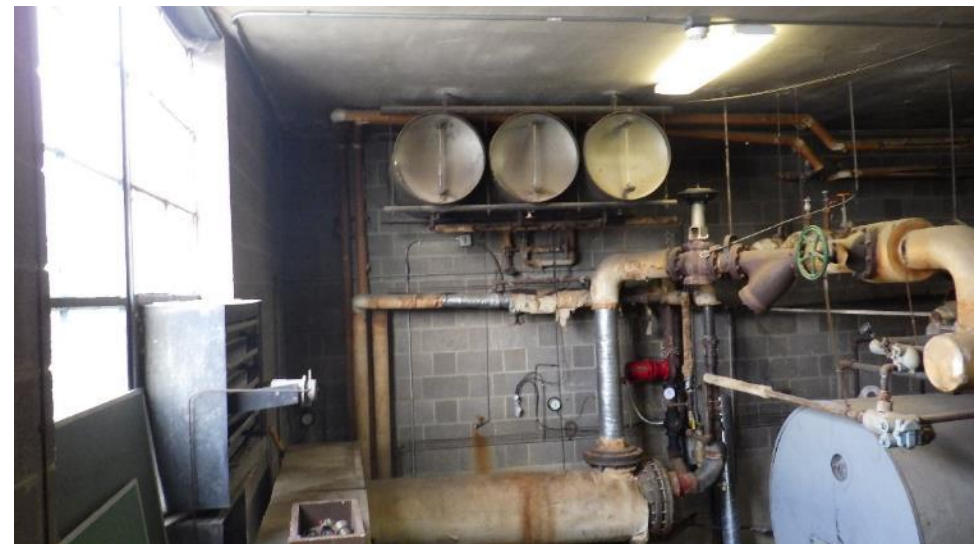
Piping with missing insulation.
