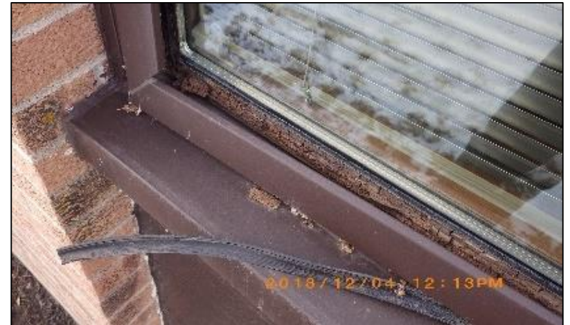
Rotted Window Sashes
