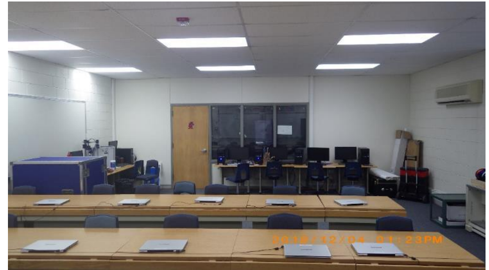
Lighting – 4-bulb T8 fluorescent troffers
