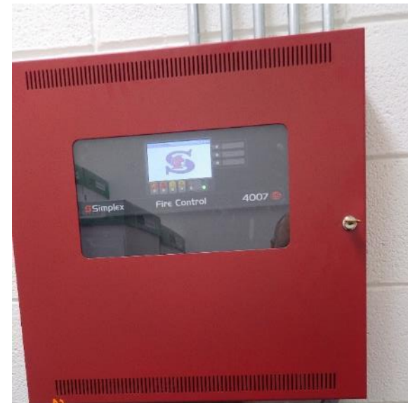
Fire Alarm (new, but obsolete)
