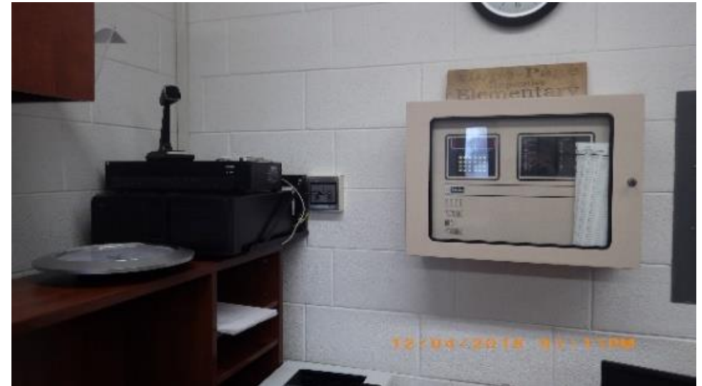
Master Clock (issues, being replaced)
