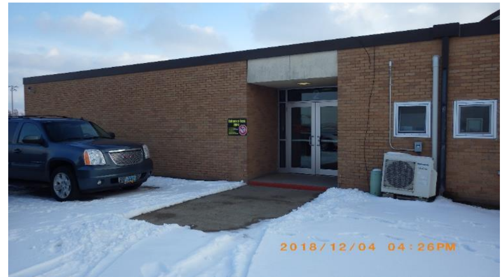
Step at Stoop, Condenser on blocks
