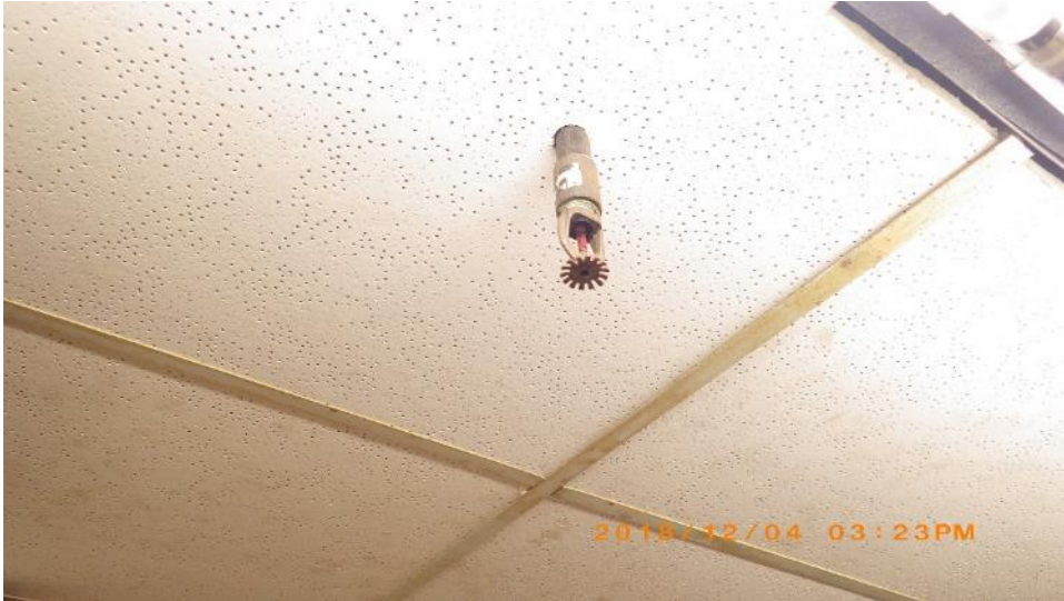
Limited Fire Suppression System
