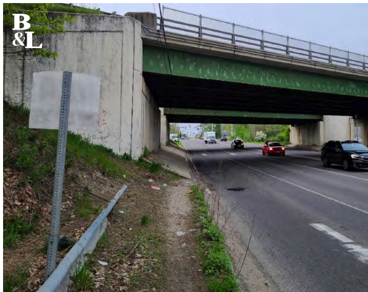
Figure 18 - Worn Pedestrian Foot Path on Payne Road
