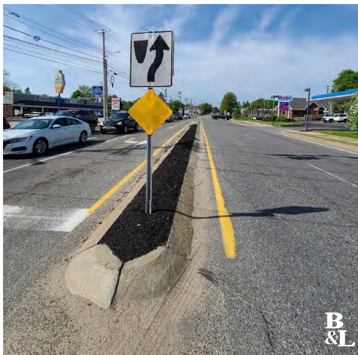
Figure 9 - Segment of Route 1 from Broadturn Road to Dunstan Avenue, Street View Facing South
