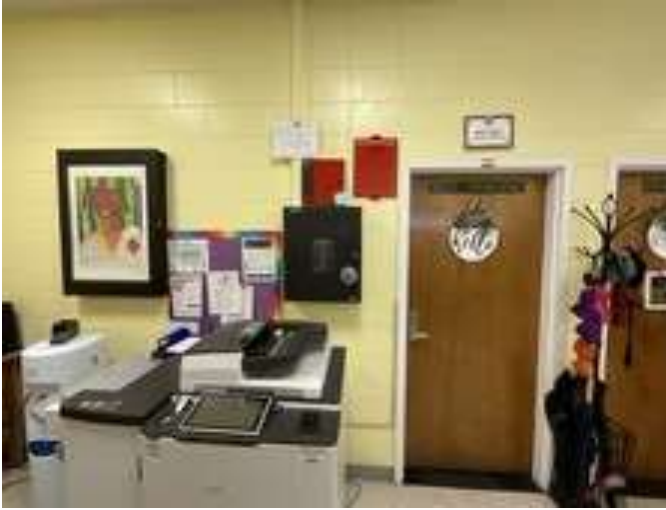
23 - FIRE ALARM PANEL
