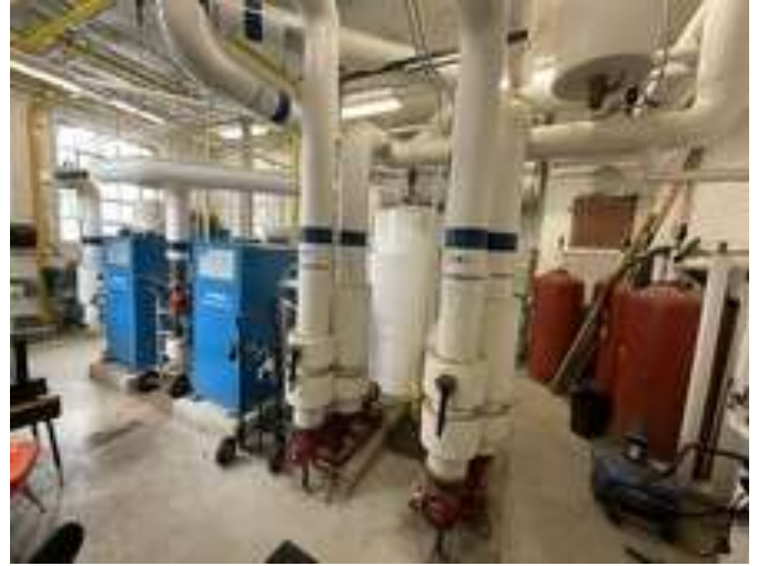
18 - MAIN MECHANICAL ROOM
