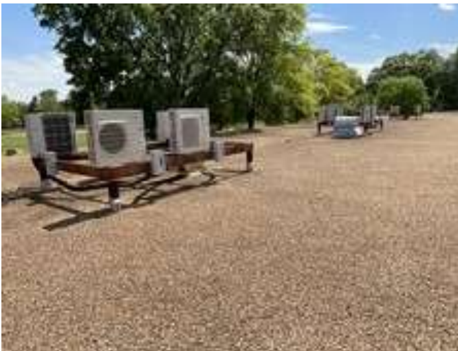
19 - ROOFTOP MECHANICAL EQUIPMENT
