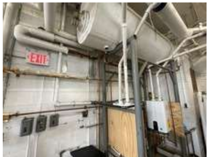
16 - DOMESTIC WATER PIPING
