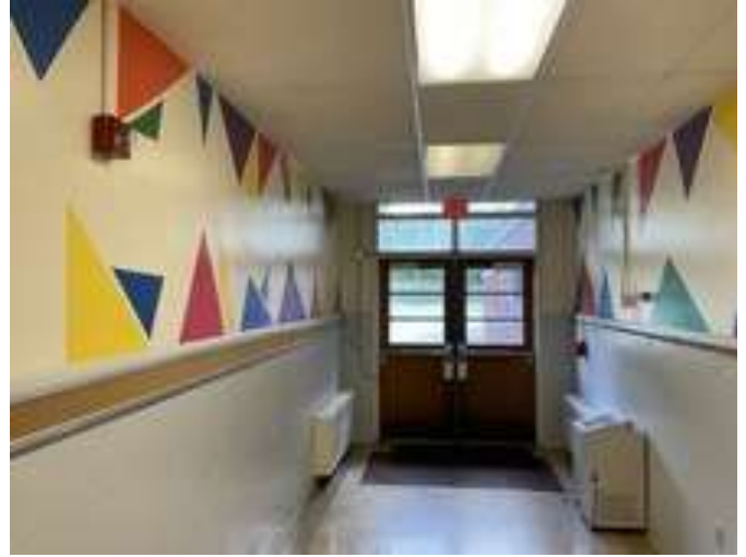
24 - FIRE ALARM DEVICES
