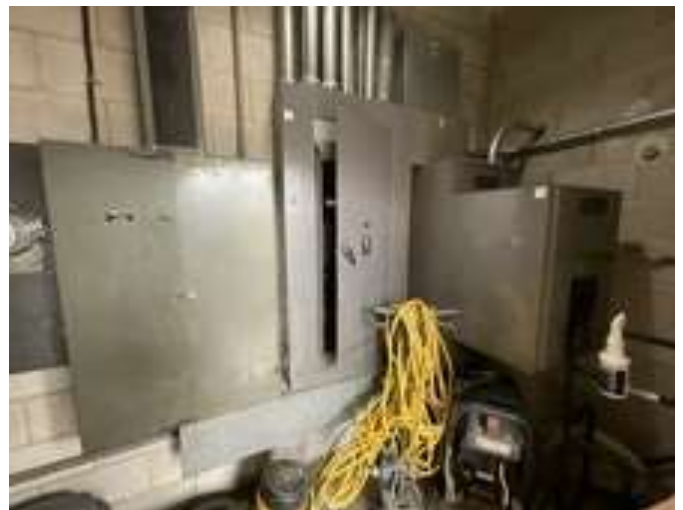
22 - MAIN ELECTRICAL ROOM
