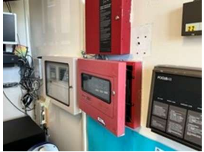
12 - FIRE ALARM CONTROL PANEL
