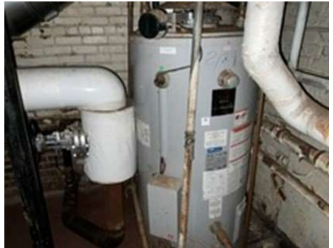
8 - DOMESTIC WATER HEATER
