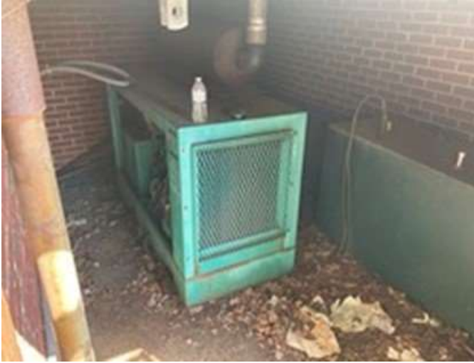
11 – EMERGENCY BACKUP GENERATOR
