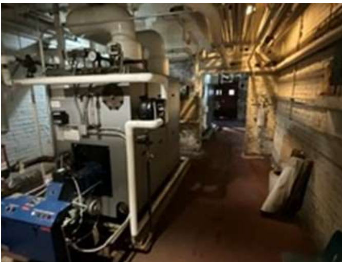
9 - MAIN MECHANICAL ROOM - HVAC BOILERS
