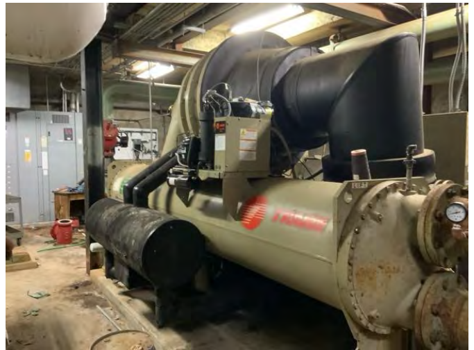
10 - MECHANICAL ROOM - CHILLER
