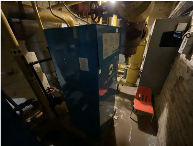
9 - MECHANICAL ROOM - HVAC BOILER
