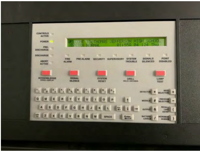
15 - FIRE ALARM PANEL
