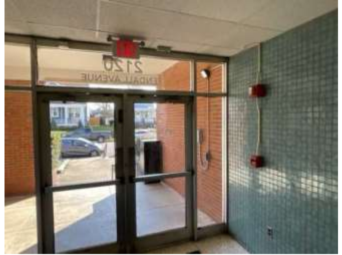
18 - FIRE ALARM SYSTEM COMPONENTS
