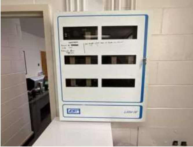
17 - FIRE ALARM PANEL
